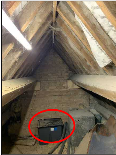
Photo 9 Location of bat droppings
