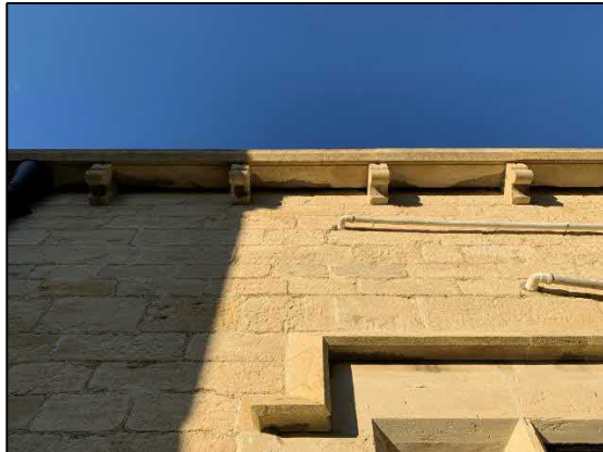
Photo 5 Gaps beneath gutters
