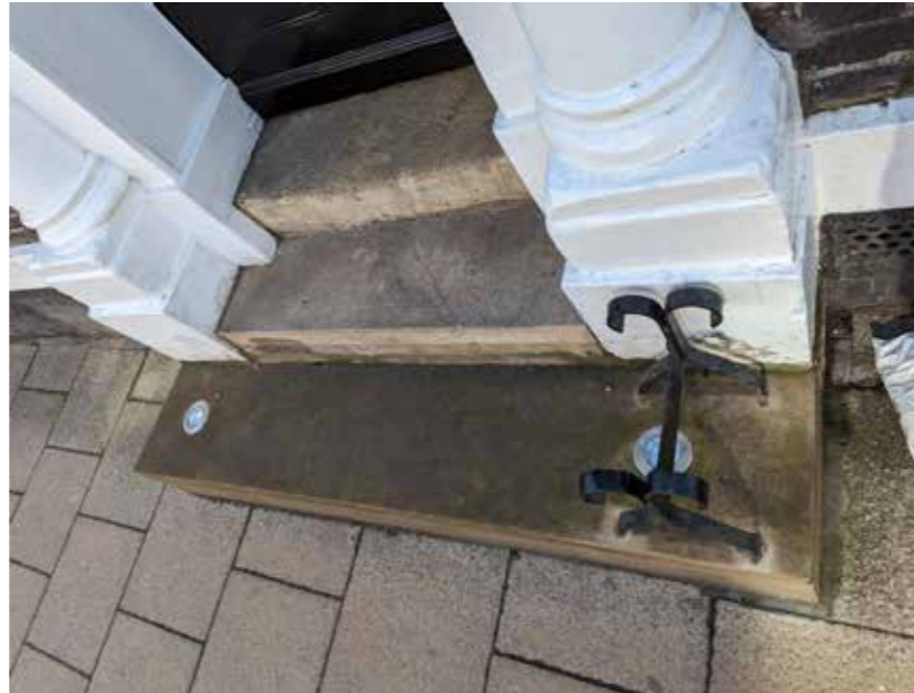
Image 2 - Current steps after repairs, showing the altered step design, new LED lights and boot scraper.
