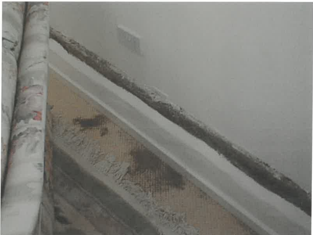
Soleplate to Outbuilding showing bore dust (South wall)
