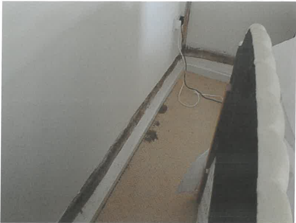
Soleplate to Outbuilding showing bore dust (East wall)
