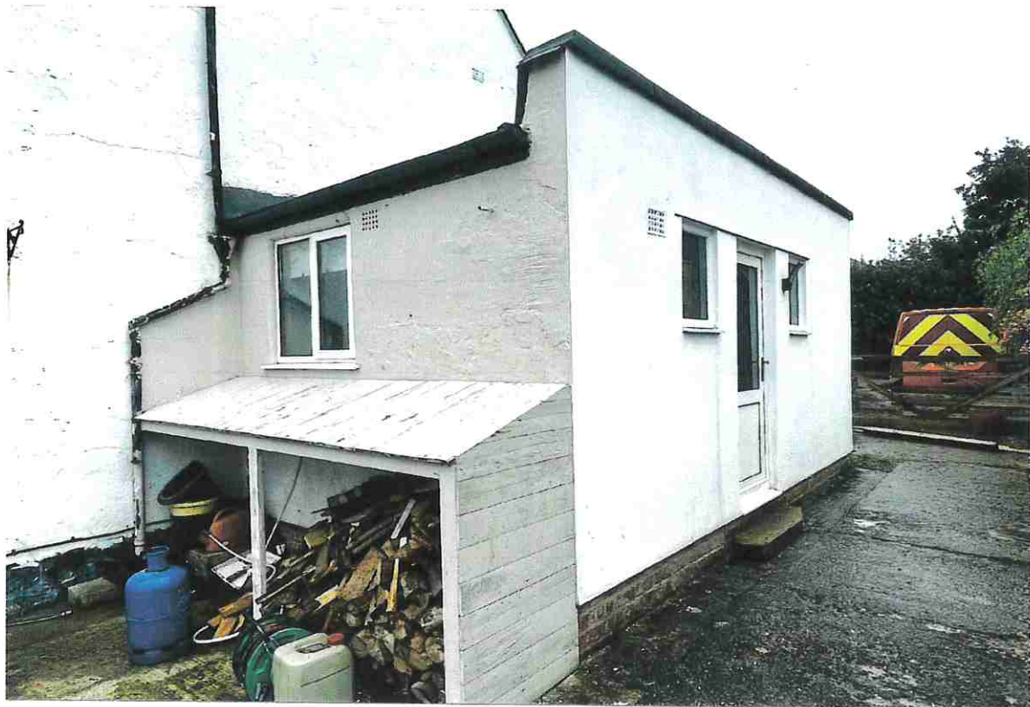
PHOTOGRAPH 3 - DETAIL OF THE SINGLE STOREY FLAT ROOF AS SEEN FROM THE REAR. IT IS PROPOSED TO CONSTRUCT A PITCHED ROOF ABOVE THE FLAT ROOF.
