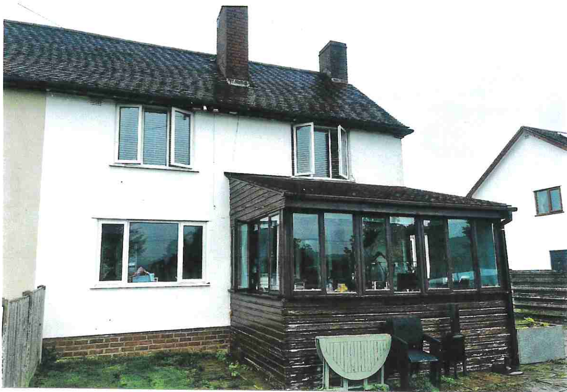
PHOTOGRAPH 5 - GENERAL VIEW OF REAR OF THE PROPERTY WHICH SHOWS THE EXISTING CONSERVATORY WHICH IT IS BEING PROPOSED TO REPLACE WITH A NEW EXTENSION.
