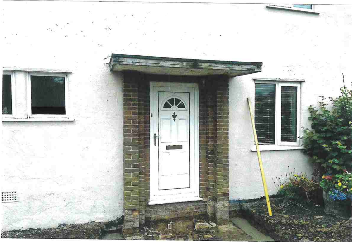
PHOTOGRAPH 8 - DETAIL OF THE ORIGINAL DOOR CANOPY. THIS IS TO BE REPLACED WITH A NEW OPEN PORCH WHICH IS SHOWN UPON THE ATTACHED DRAWINGS.
