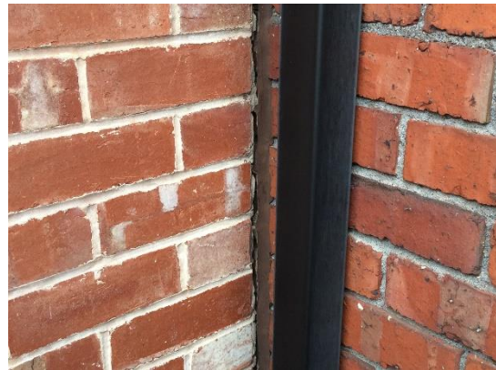
Picture 2: Rear extension/ house cracking
