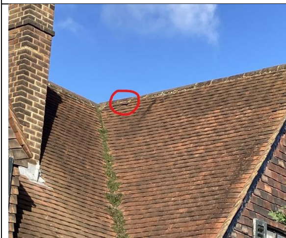
Photograph 3: Missing tile on south-east side of gable
