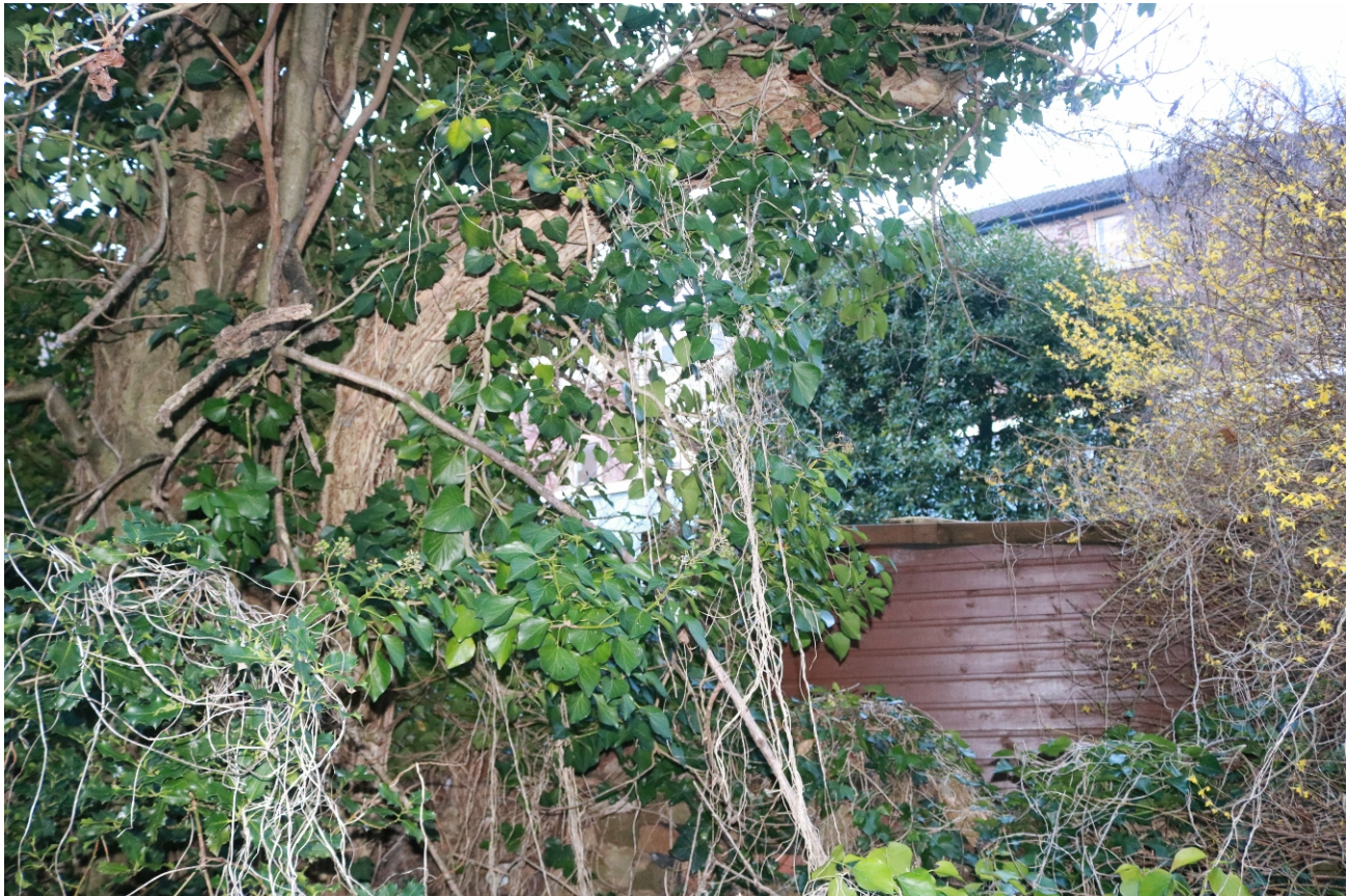
South West end of garden at ground level, March 2024 . Right hand trunk stem direction in particular worrying (see also next frame) . Shed is in adjacent property #4, to south. Green Foliage is Ivy and Holly.
