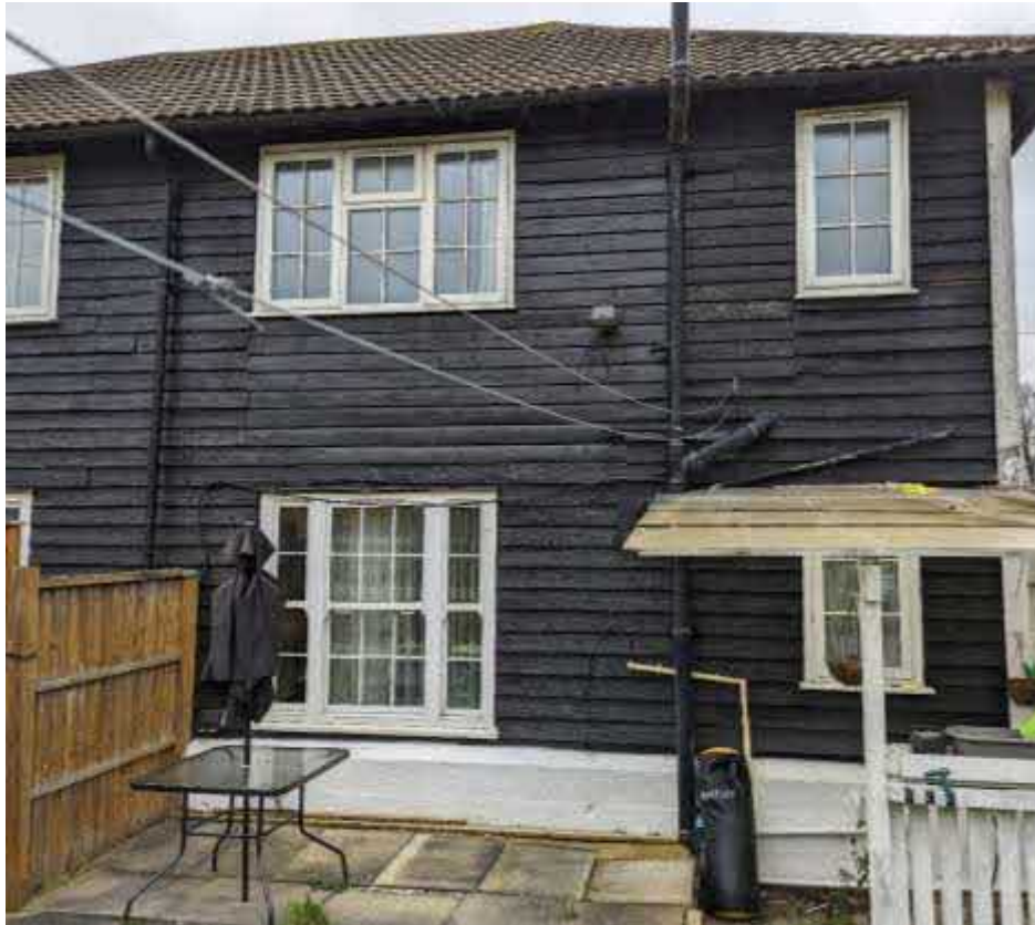
Fig. 17: Rear of 38-40 Playfield with rendered dwarf wall painted white which EWI will replicate.
