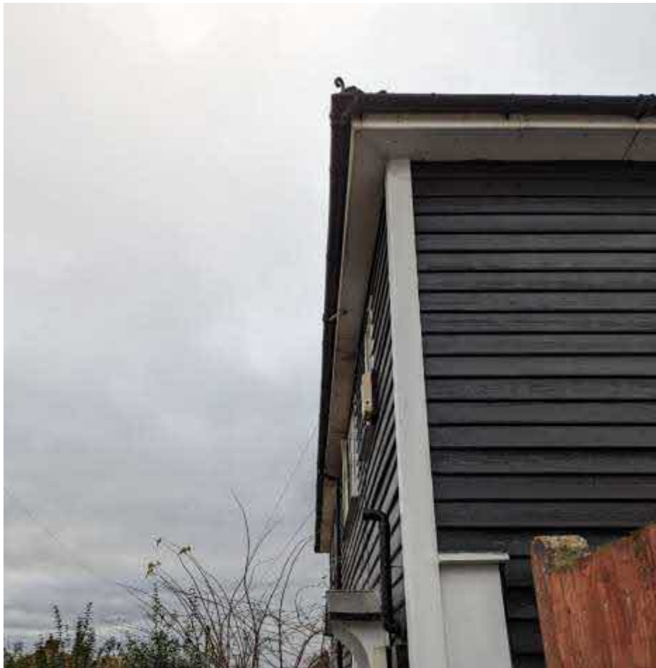
Fig.14: Deep eaves overhang allows the building line to be extend by 50mm without compromising the traditional appearance.
