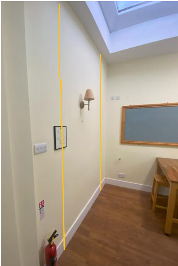
Fig 3 - Section of wall in “back” room affected by removal of “infill” section in adjacent room
