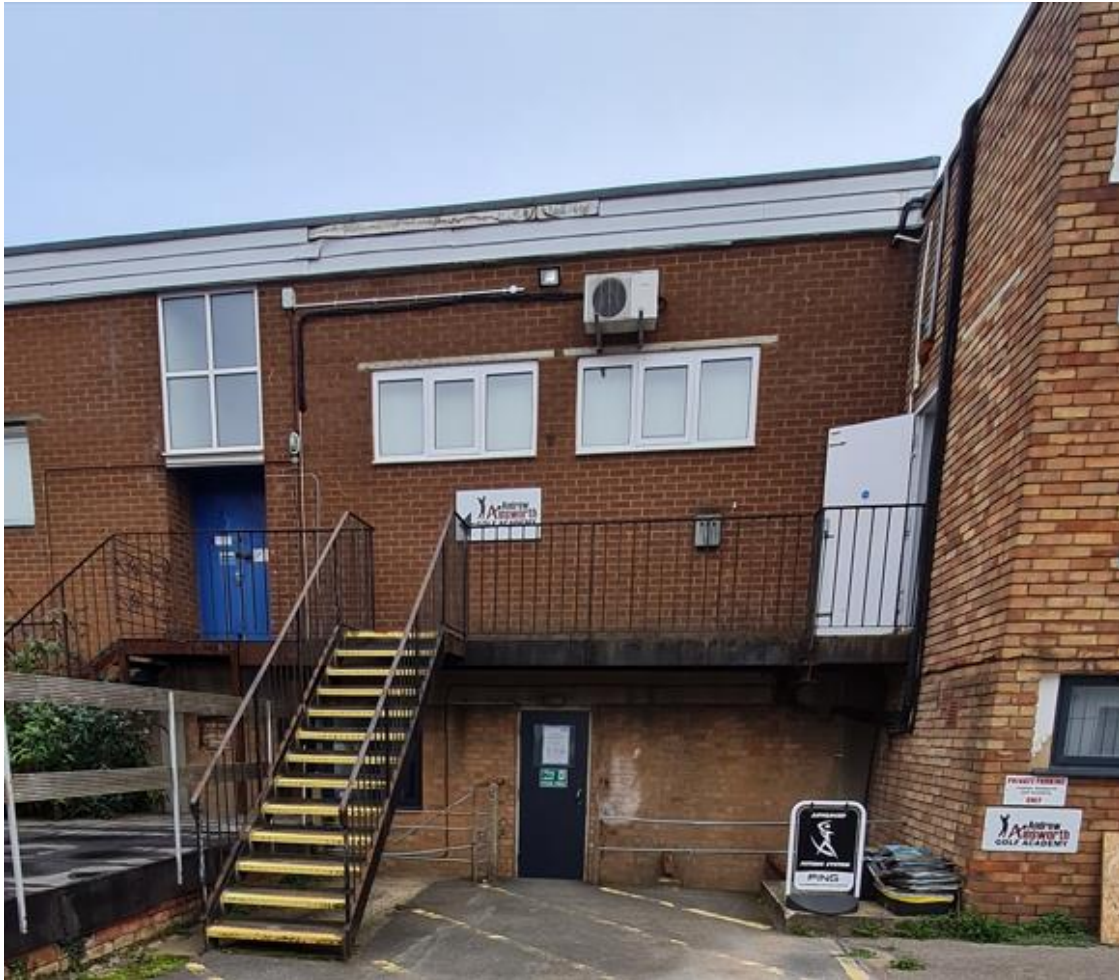
Photographs taken pre-2020 showing previously existing fire escape from Honours A and Honours B.
