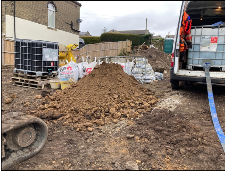
View of soil arisings from TP1 – note weathered sandstone gravel and cobbles
