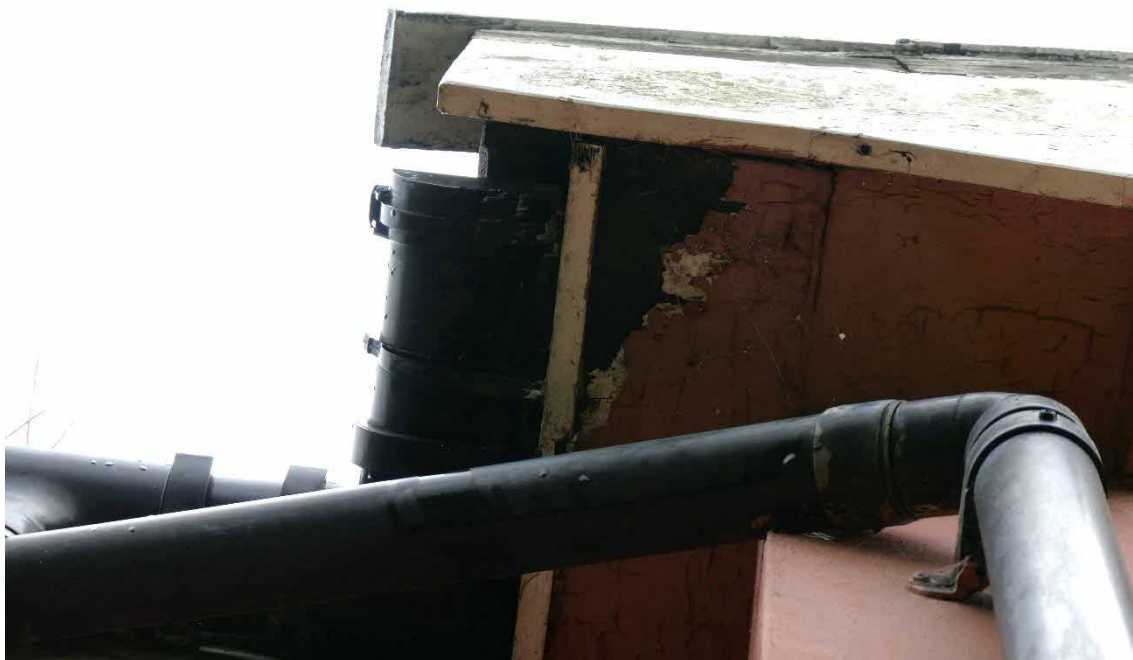
Photo 10, large gap within the soffit box at the southeast corner of building one.
