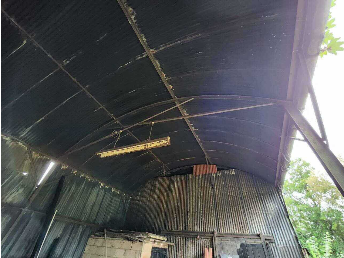
Above: Single skin corrugated profile metal sheeting roof supported on purlins/trusses/internal gable.
