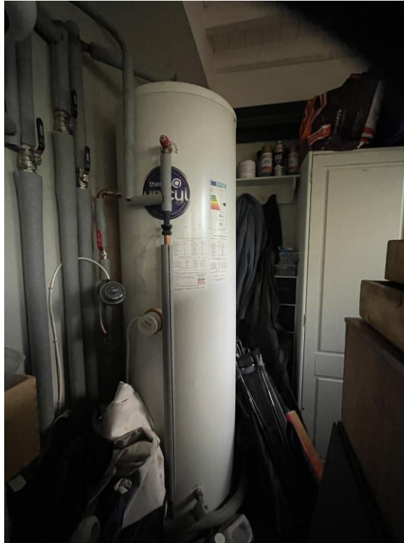
Fig.10 proposed location for the unvented hot water cylinder within C20th garage, replacing existing cylinder..
