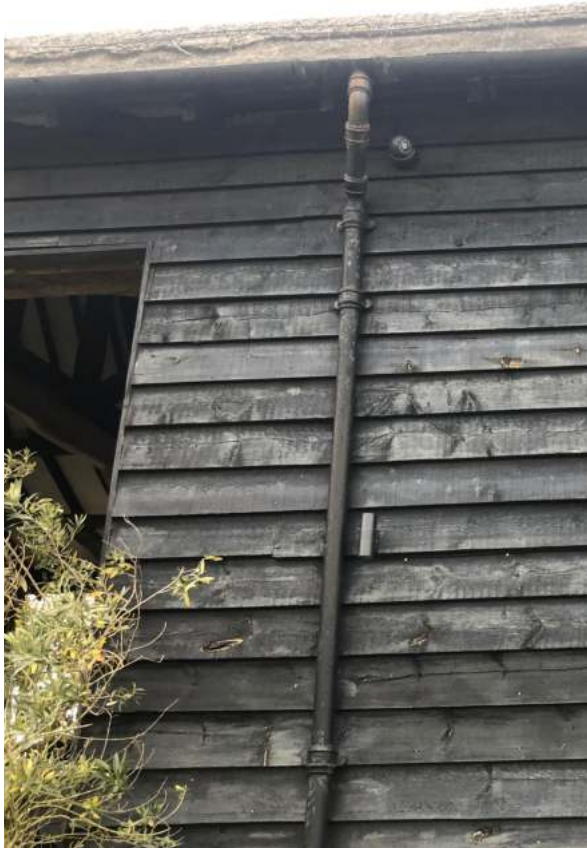
CCTV camera positioned close to domestic guttering
