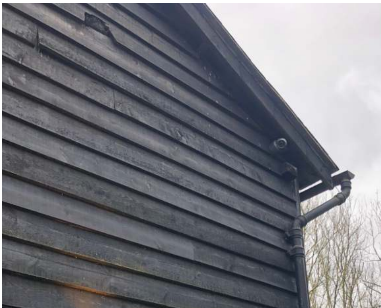
1 no. CCTV camera in situ
