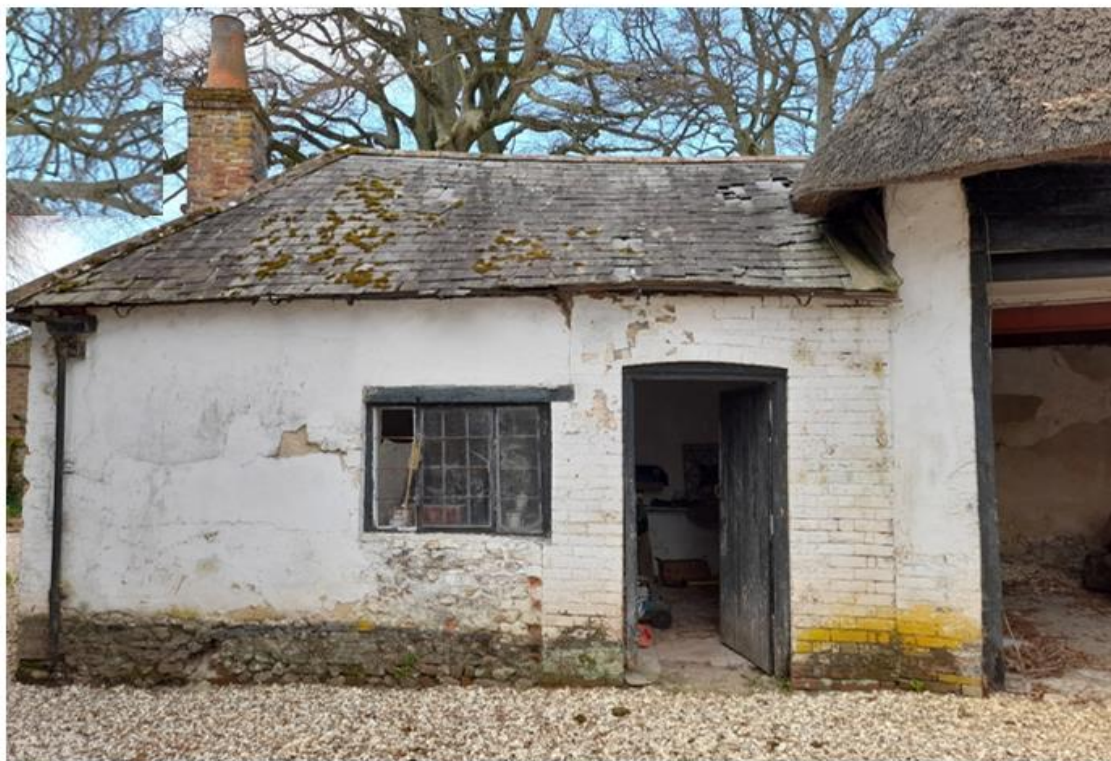
Fig. 18: View, looking west, of the small single-storey building to the left of the Coach House.
