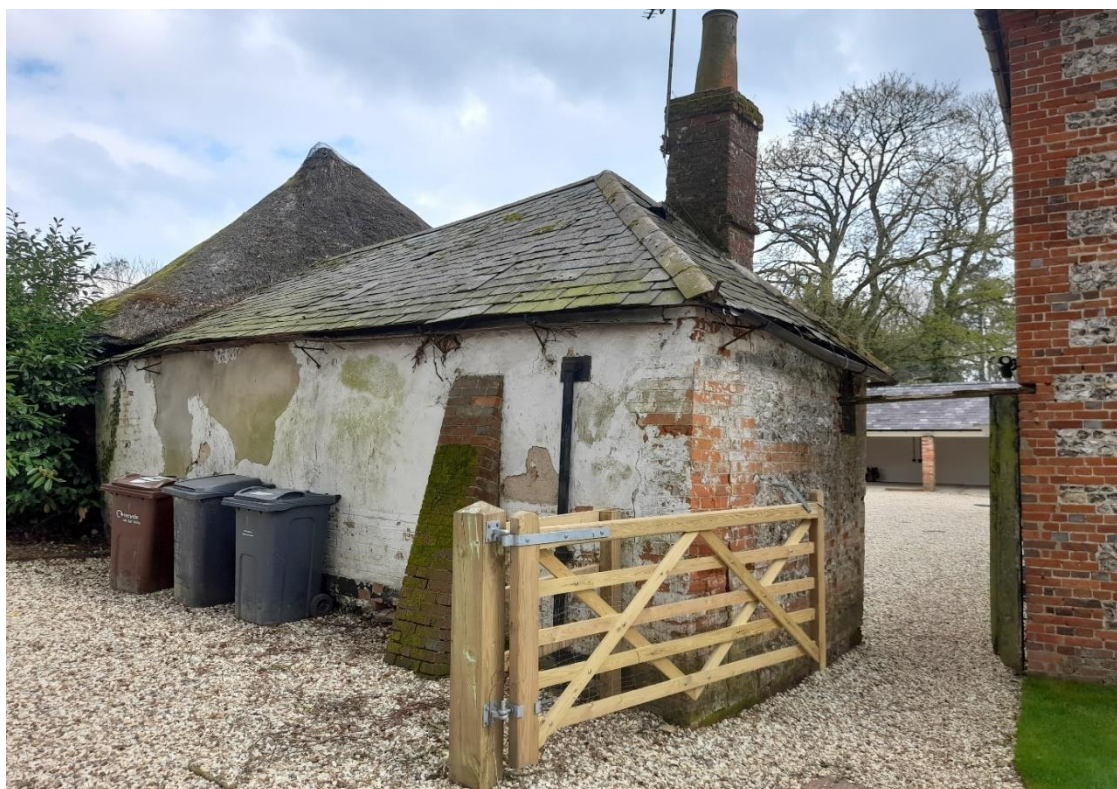
Fig. 22: View, looking north-east, with the side and rear elevations of the small, single-storey building, with details of construction.
