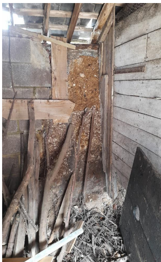
Fig. 25: Looking north within the interior of the eastern range, with cob and concrete block construction of the rear wall.
