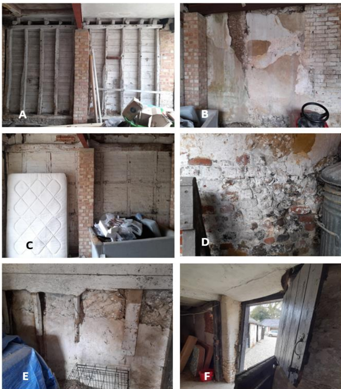
Fig. 16 A-F: Details of original fabric and construction within the central coach house.
