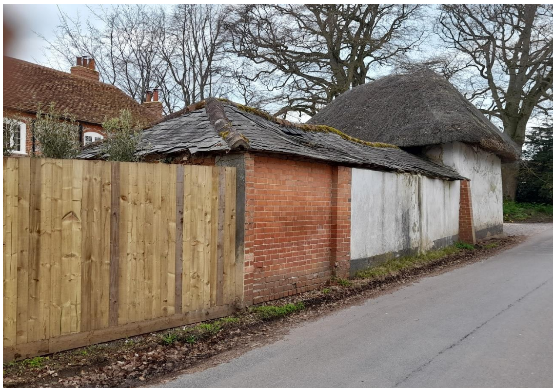
Fig. 36: View, looking south-west from Amport Road, with the existing rear elevations of the outbuildings.
