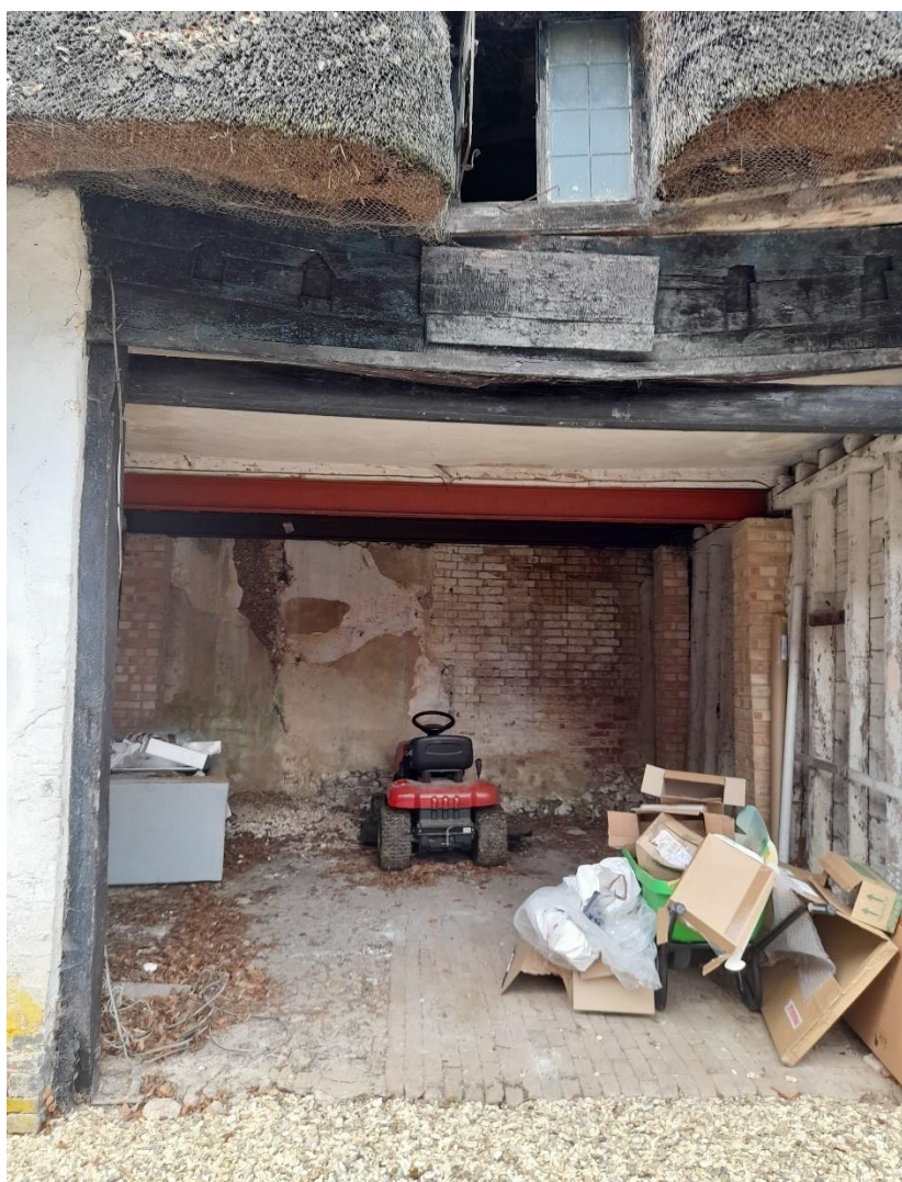
Fig. 13: View, looking west, of the coach house entrance, with details of internal construction and recent repair.
