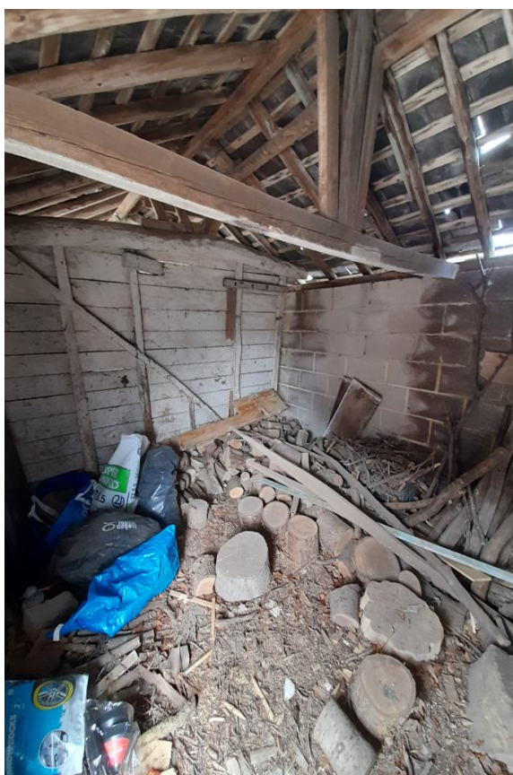
Fig. 24: Looking north-west within an interior space within the eastern single-storey range, with details of roof construction and timber partition.
