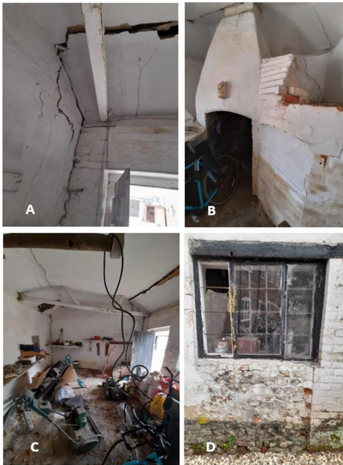
Fig. 21: A-D: Details of internal and external features of the small, single-storey building to the left of the coach house.
