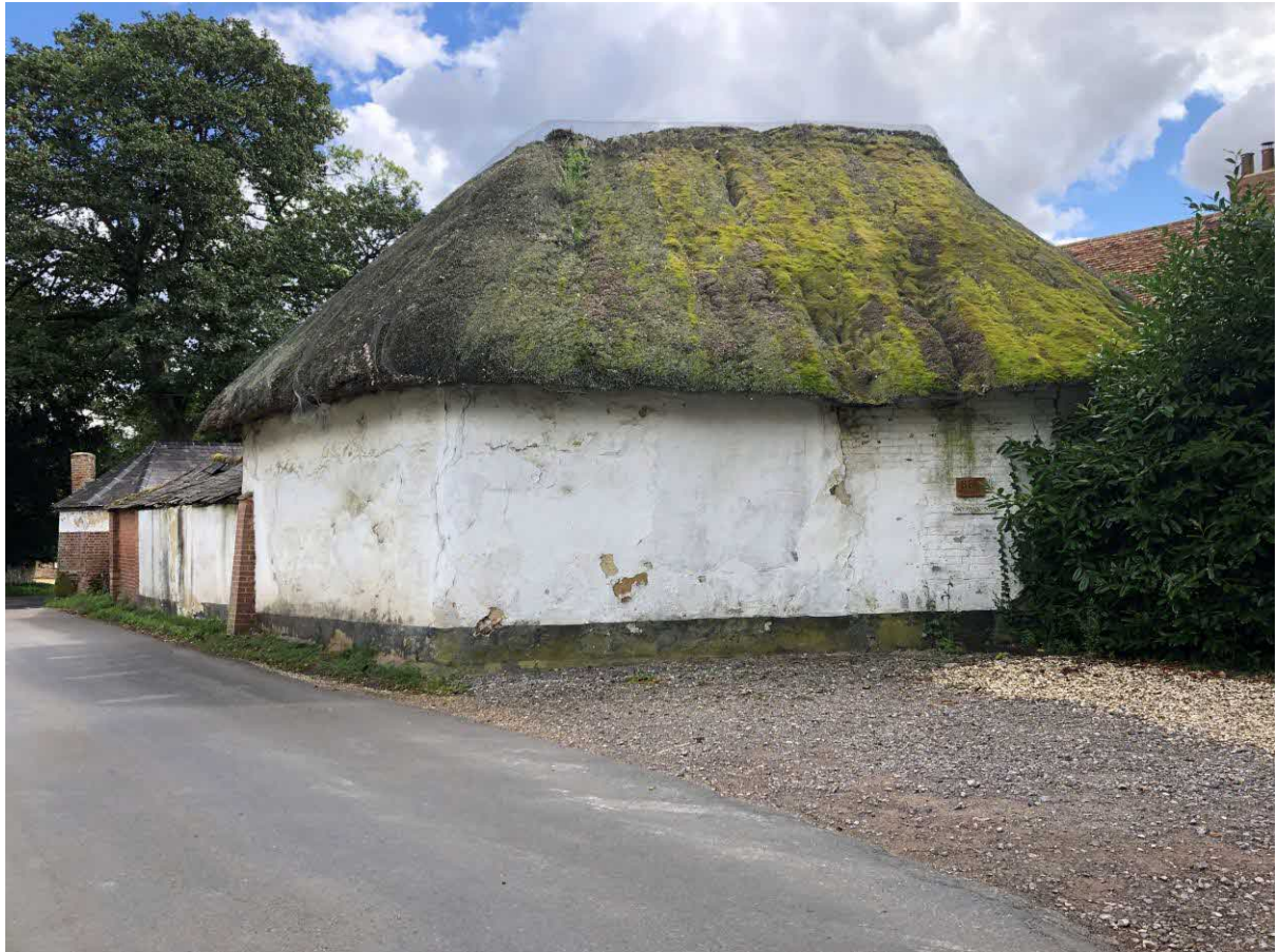
External General View of Coach House Stable Rear Wall – Note Small Roadside Buttress and Coach House Brick Patch to the right
