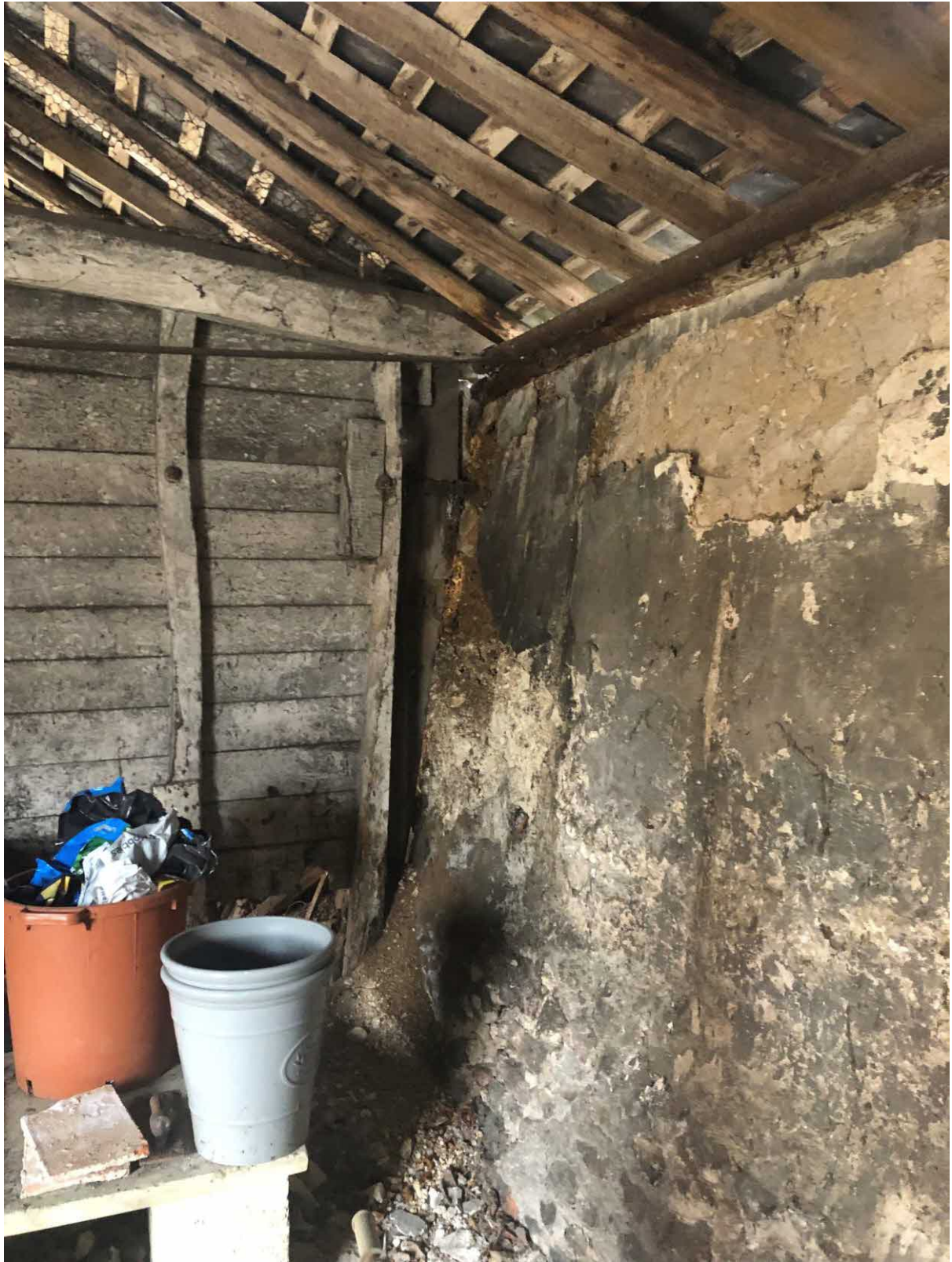
Stables Road Side Wall - Note Leaning Outwards Cob Wall
