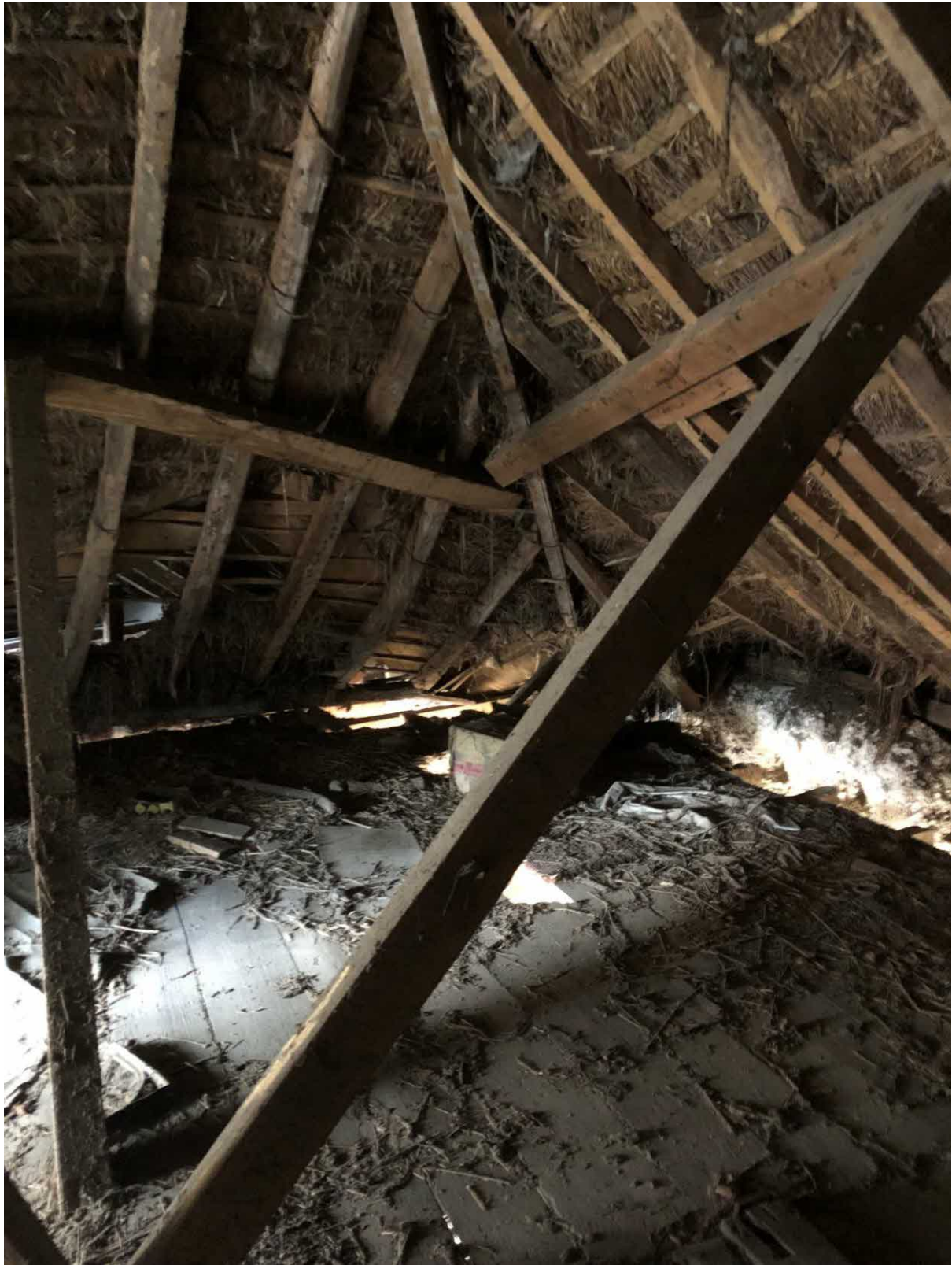
View of Coach House Roof Structure Looking Towards Bothy and Rear Elevation – note roof spread at eaves
