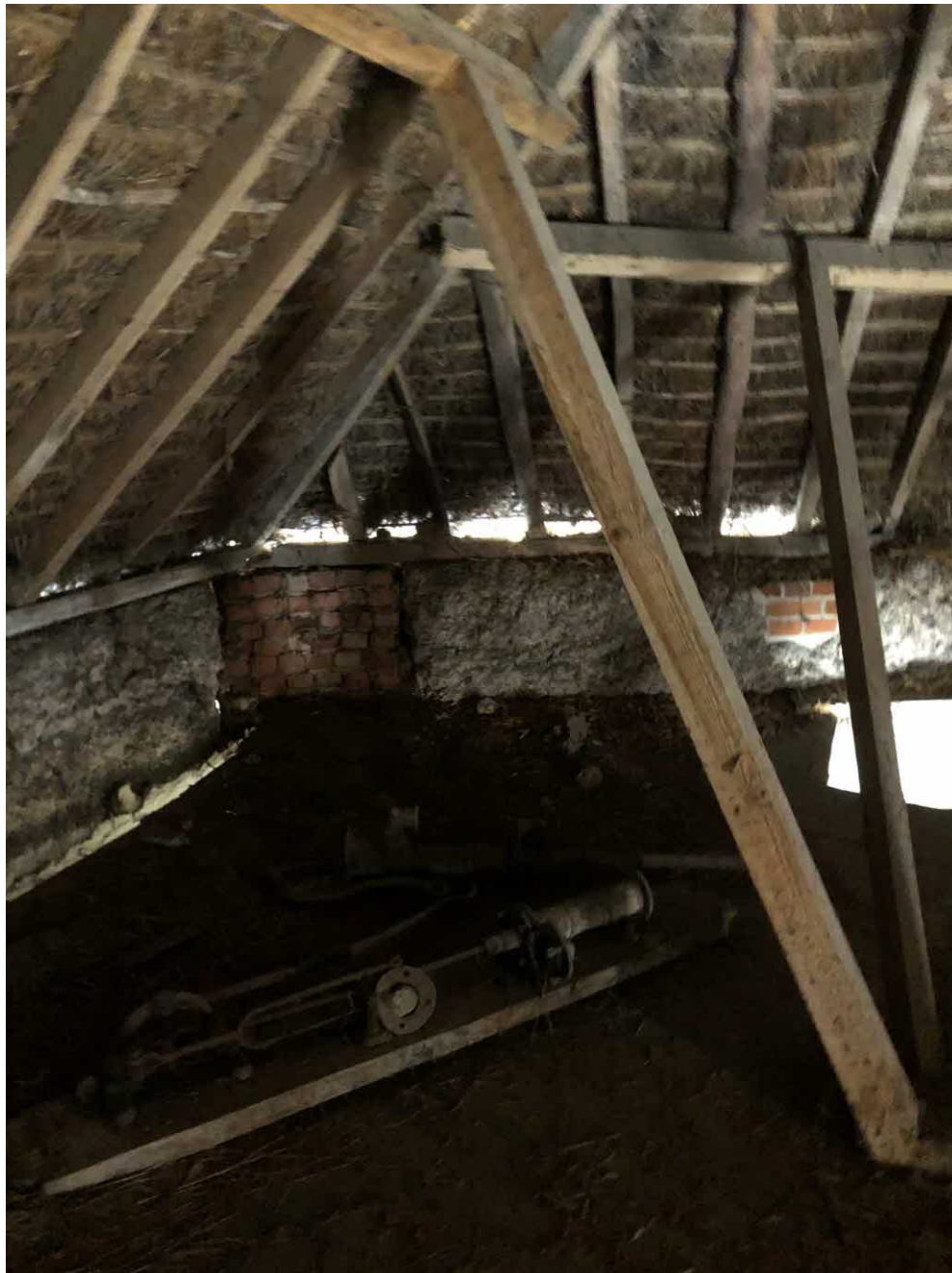
Later Strutting and Purlins in the Stable Area of The Coach House Roof – note Outward Leaning Walls
