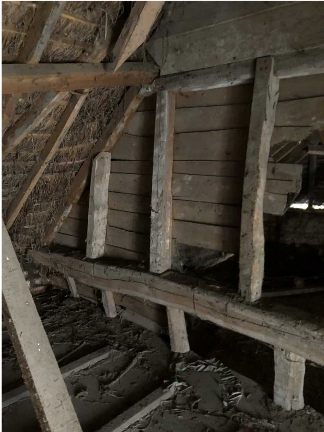
Note Boarding on Former Gable Wall Between Coach House and Stable
