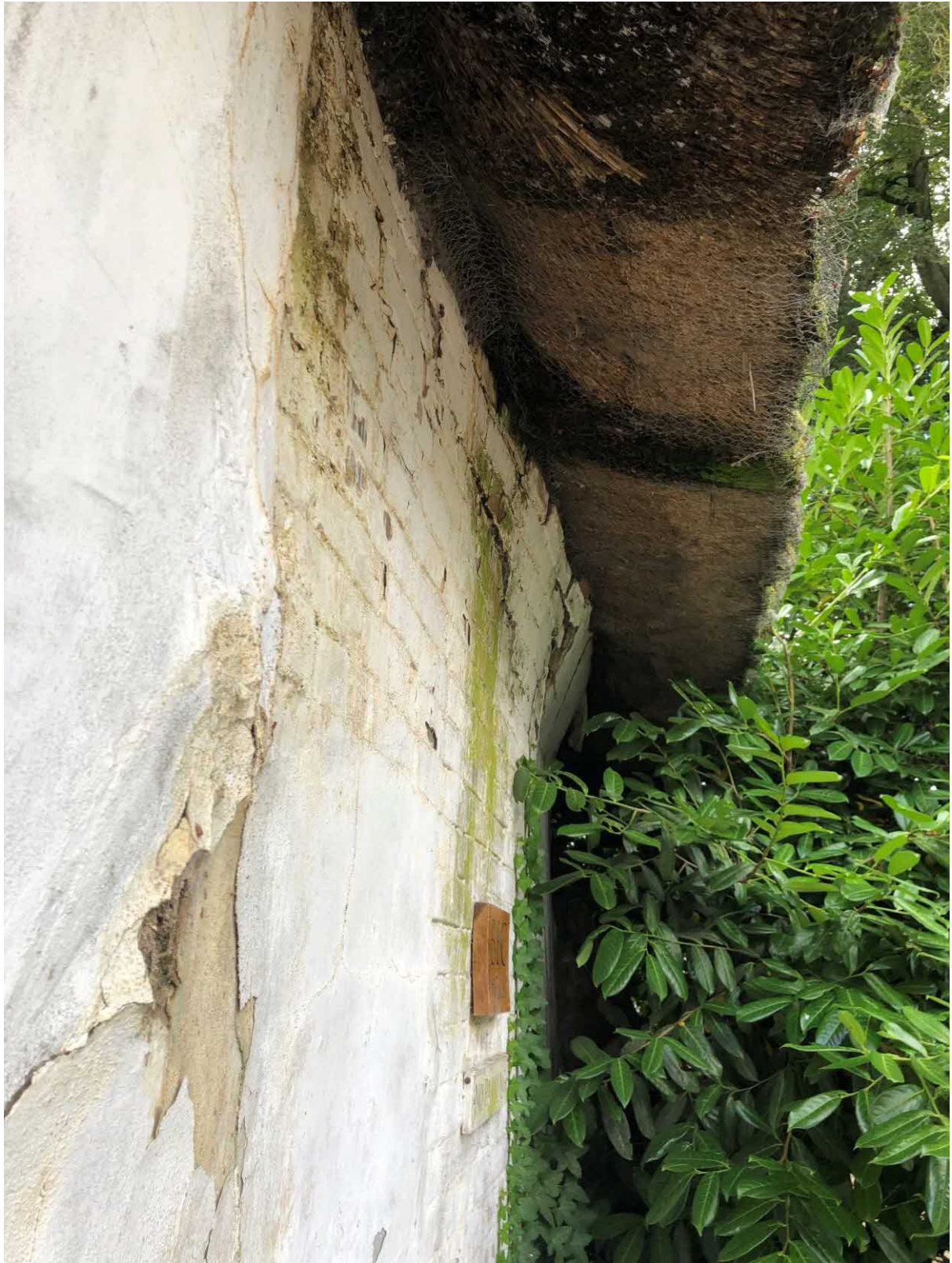
Note Outward Lean of Coach House Rear Wall Brick Patch – Very Unstable
