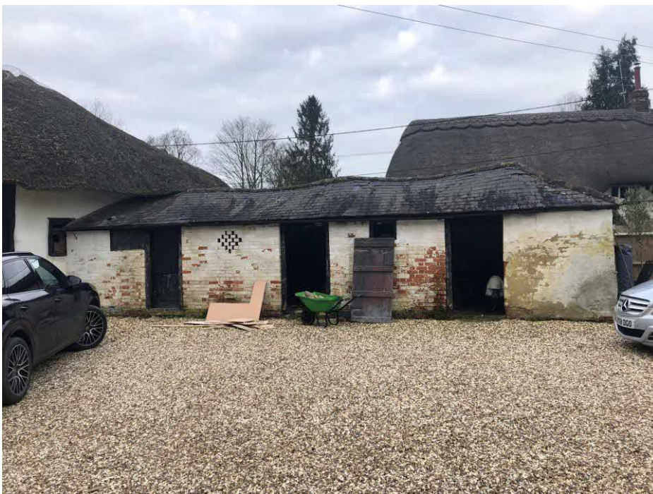
View of Stables Yard Side Elevation – Note Failed Roof.
