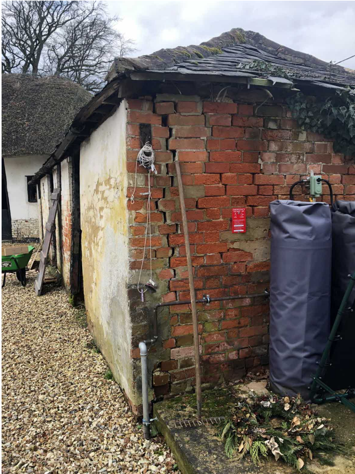
Stables Yard Side Wall – Note Outward Lean and Cracking with return wall (also uneven failed roof structure)
