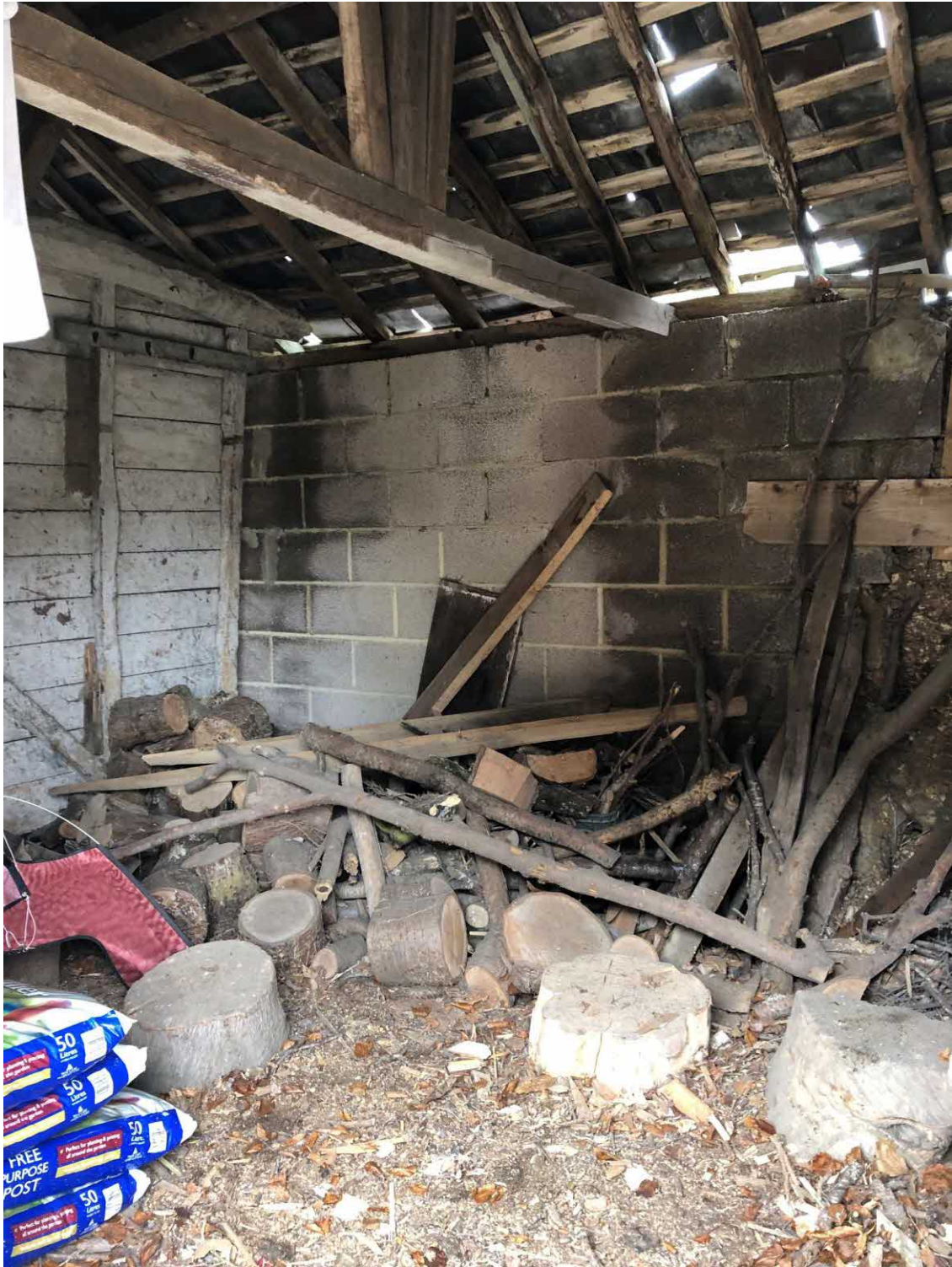
Stables Road Side Wall – Note Modern Concrete Block Replaced Section ( Where Original Cob Has Collapsed)
