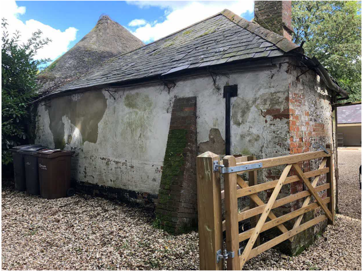
External General View of Bothy Rear Wall – Note Historic Buttress and dark rendered Brick Patch
