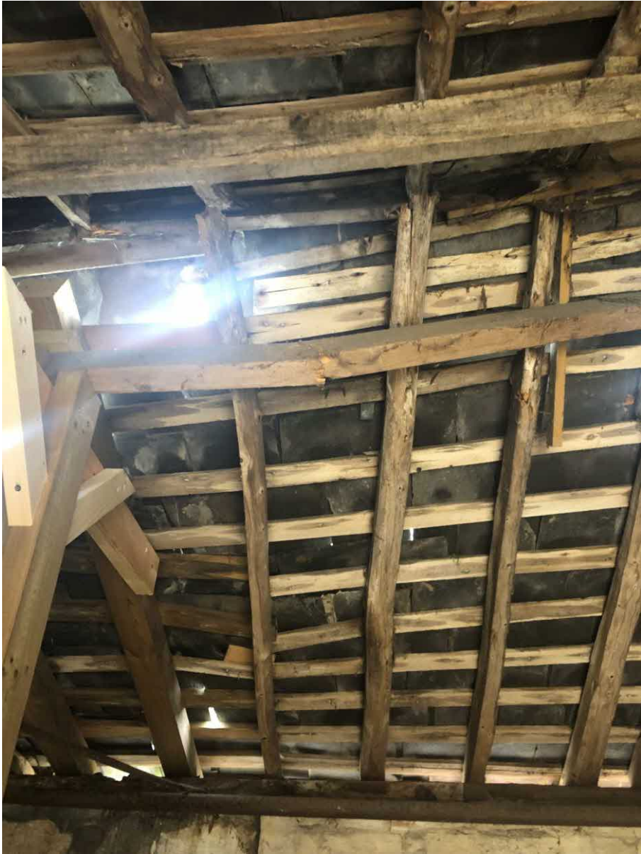
Stables Roof – Note Broken Purlin and Detached Rafter From Ridge
