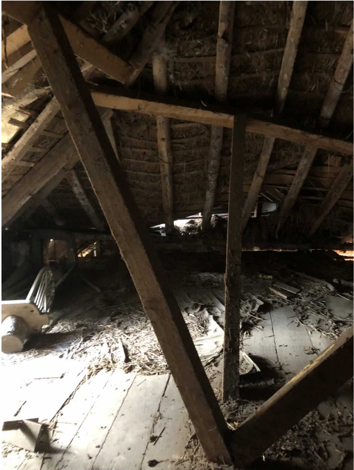
View of Coach House Roof Structure Looking Towards Bothy – note later purlins and strutting
