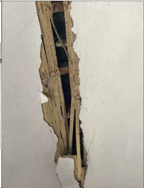
Photograph 10: Hole into roof space.(A)
