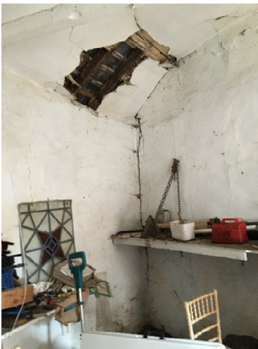
Ceiling cracks and plaster falling in
