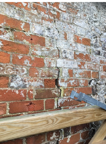
Cracks in brickwork on Bothy building
