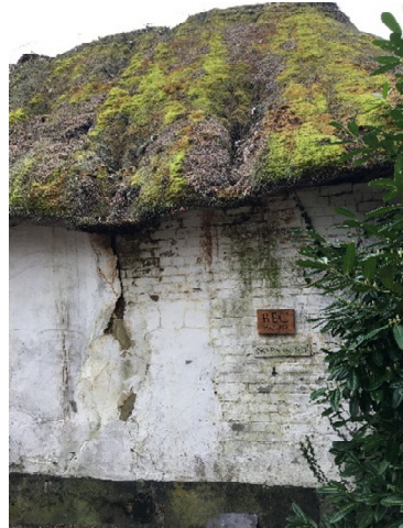
Thatch failing and allowing water into fabric
