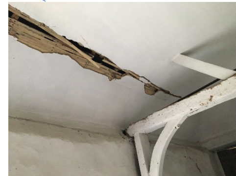
Ceiling cracks and plaster falling in
