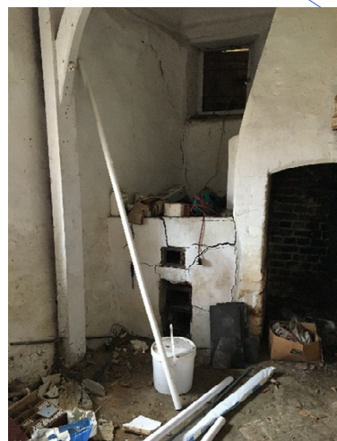
Cracks in oven/fireplace feature
