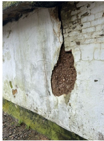
Cobb damage due to water ingress
