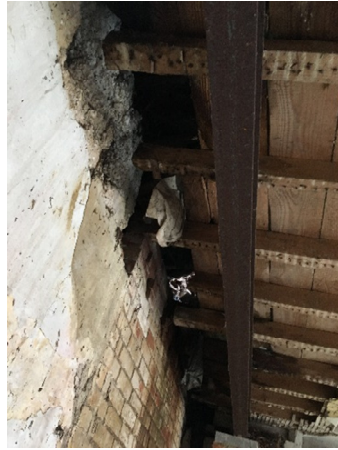
Floor joists coming away from wall
