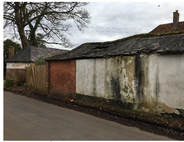
Stable roofs have failed and are falling inwards
