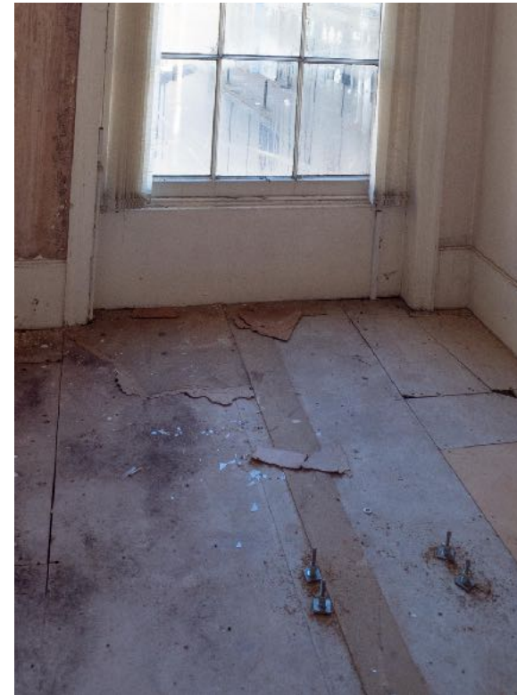
Existing kitchen hood fixings to be removed and hood re fixed to ex kitchen ceiling.
