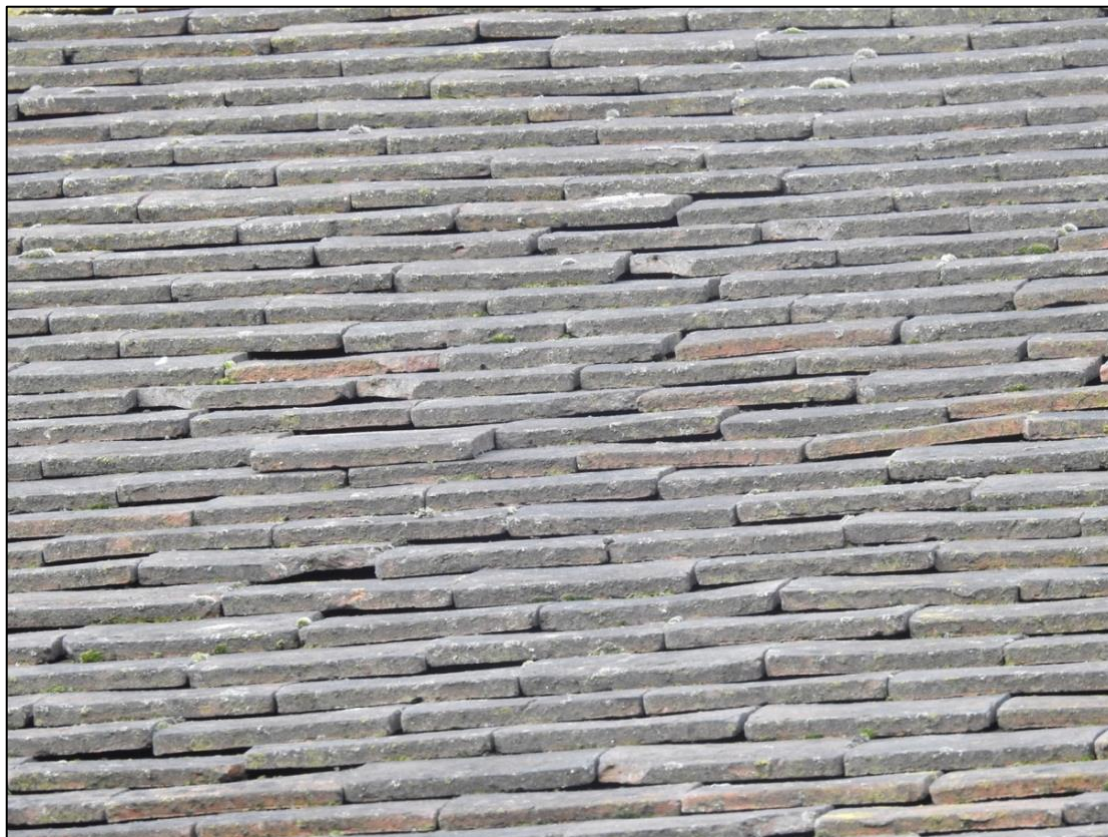
Photograph 9. Showing an example of gaps between slipped and raised roof tiles.
