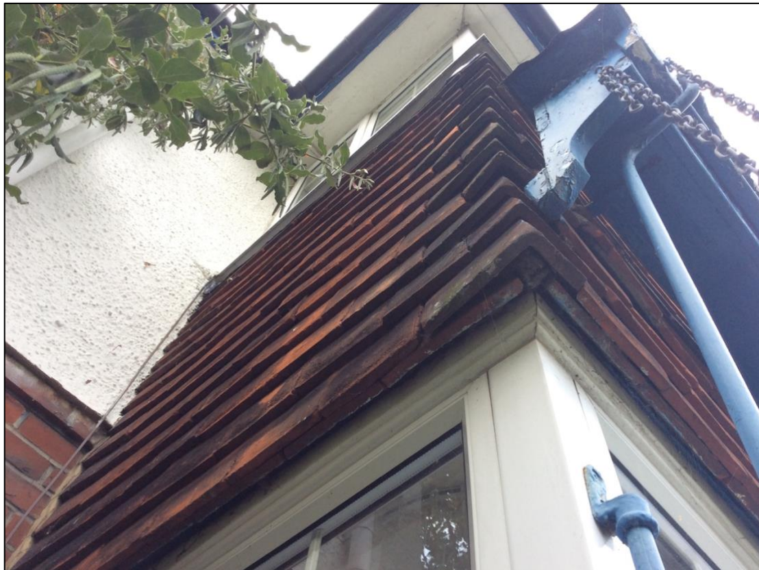
Photograph 12. Showing an example of gaps between hanging tiles.
