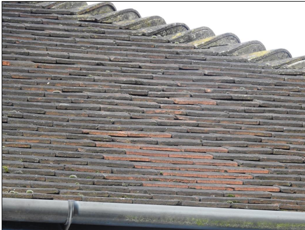
Photograph 10. Showing an example of gaps between slipped and raised roof tiles.
