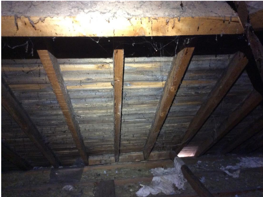
Photograph 14. An example of the gaps identified at eaves level allowing potential access by bats into the internal roof void.
