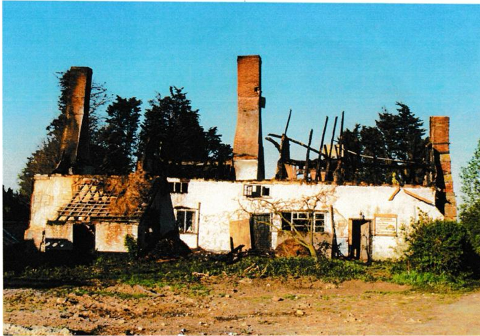
Figure 2. Historic photograph of Southwest (farmyard) elevation showing fire damage in 1980s.
