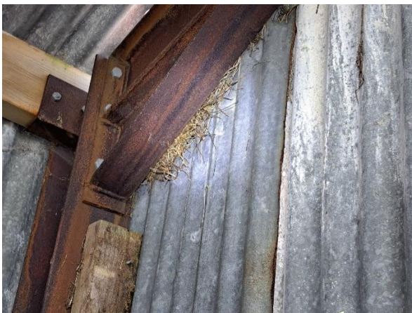
Photographs 4-6: Old bird nests associated with the barn's metal frame
