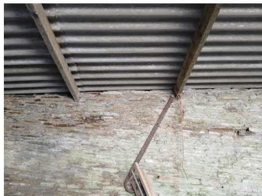
Photograph 6 – View of gaps along the wall tops.
