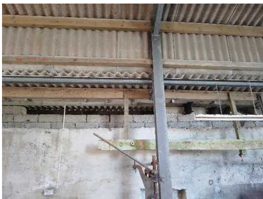
Photograph 5 – View of gaps along the joins between the roofs.
