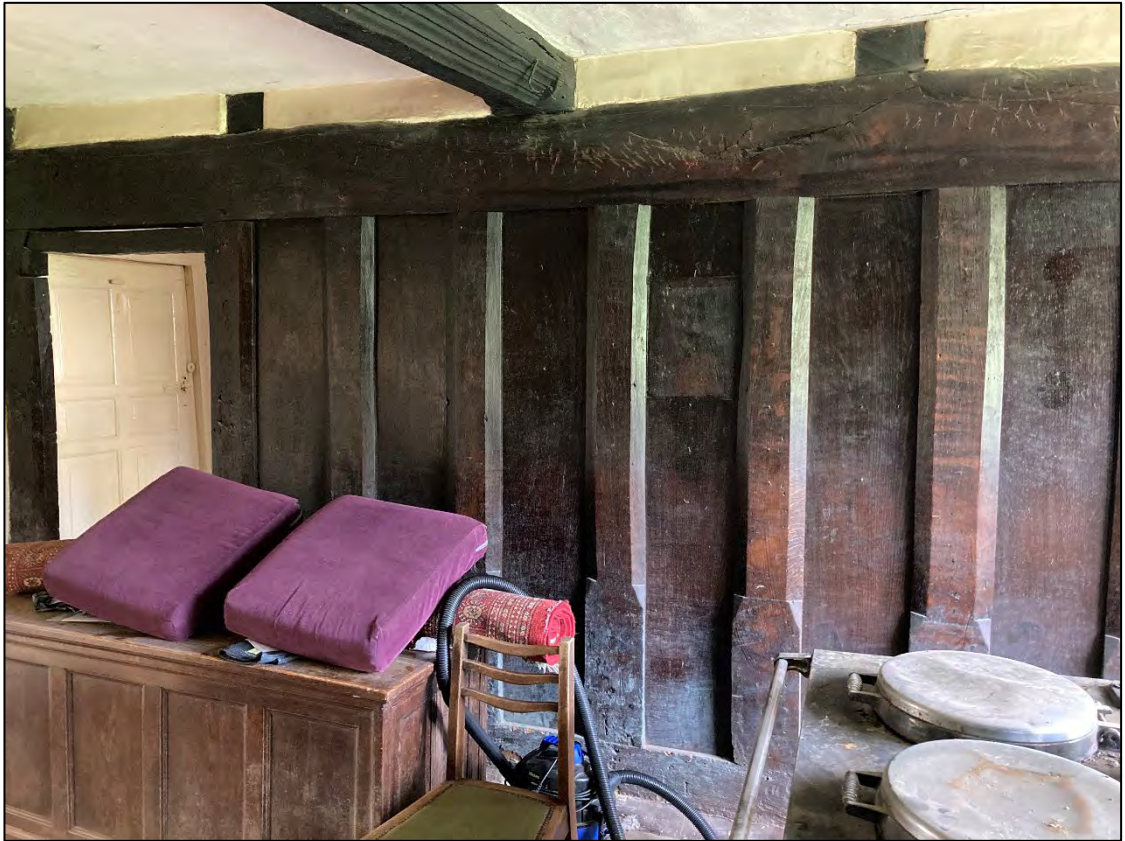
Figure 14: Oak plank-and-muntin screen separating Room 1 from Room 2. Note how the screen is installed into the large oak crossbeam running through the centre of the hall.
