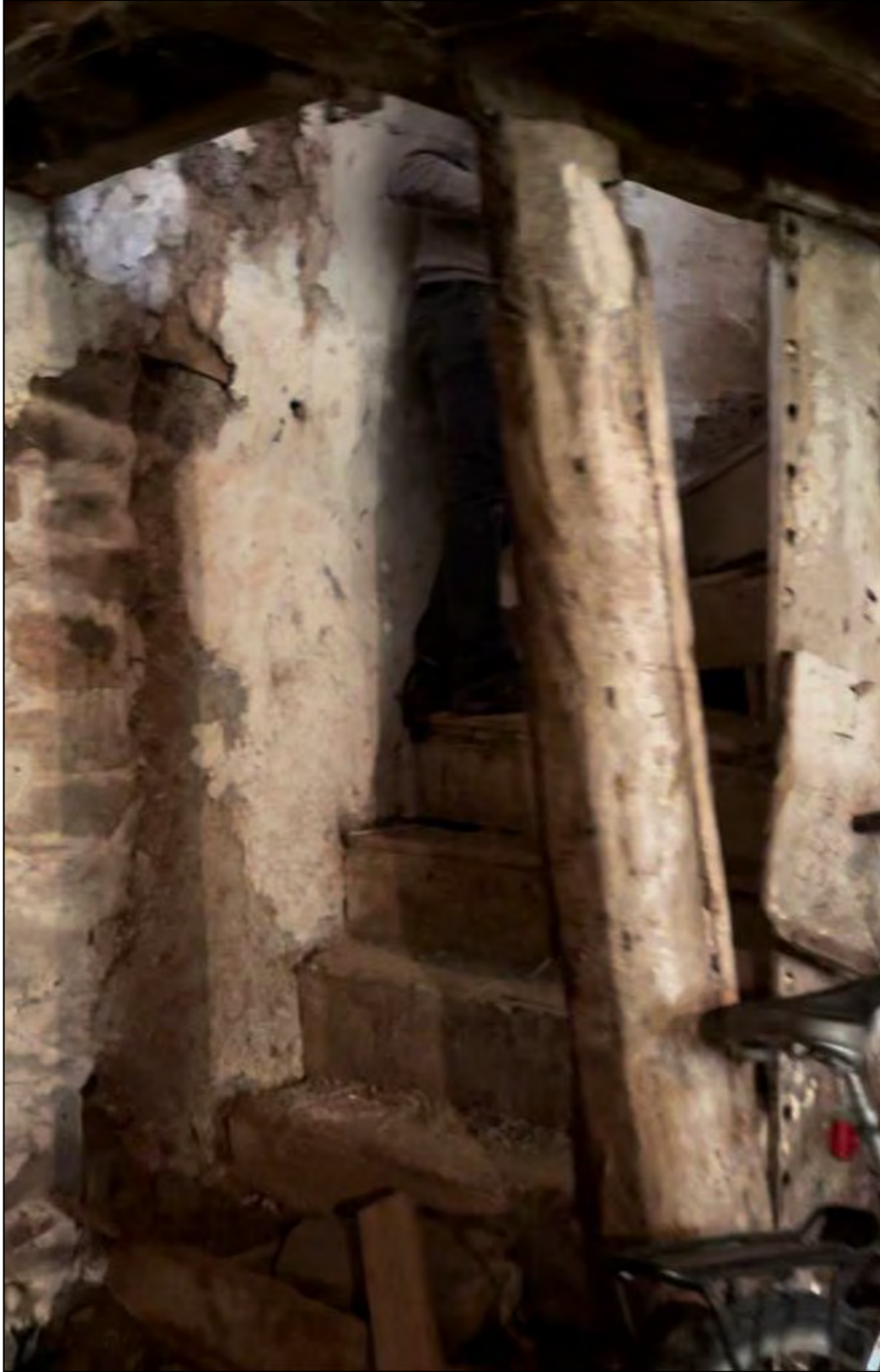
Figure 41: Staircase within Room 9. The vertical beams are likely to be original although its stairs may have been replaced.
