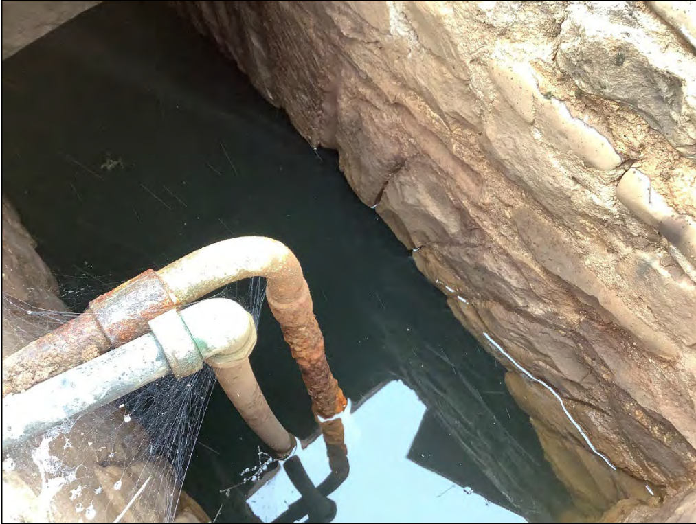
Figure 57: Cistern/well beneath the central courtyard. Its stonework is bonded with lime mortar.
