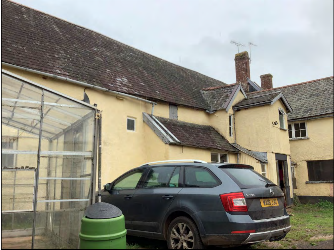
Figure 10: The southern elevation of the main block from the internal courtyard with later small lean-to porches jutting out from the main block. View to north east.
