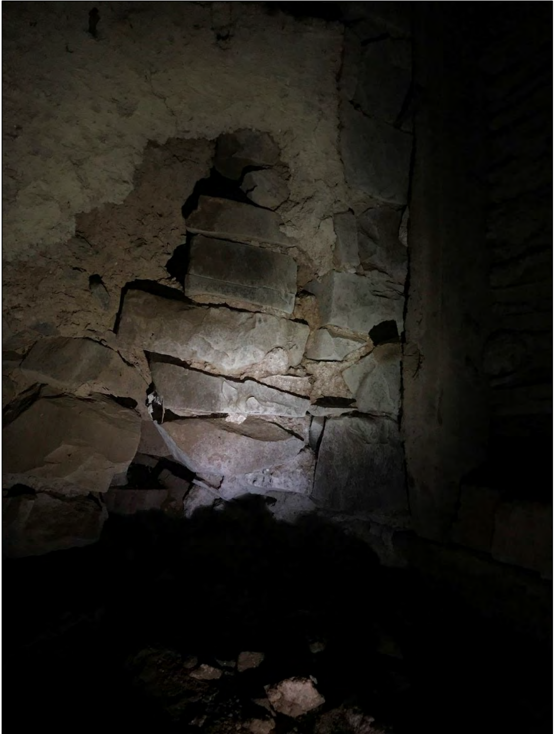
Figure 36: Cob over rubble wall to the north of Room 8 likely represents the original external wall of the hall house.
