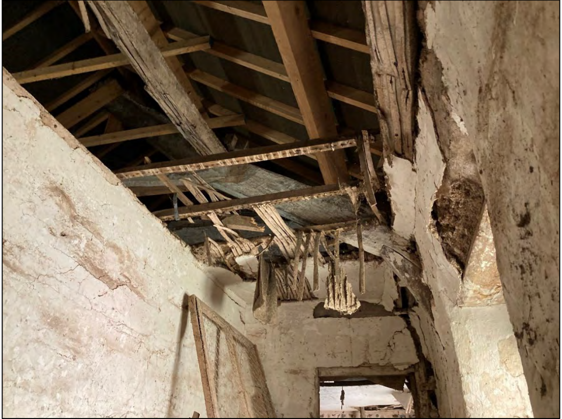
Figure 44: Roof structure of the southern block. The jointed cruck frame is overlain by a 20th century re-roofing.
