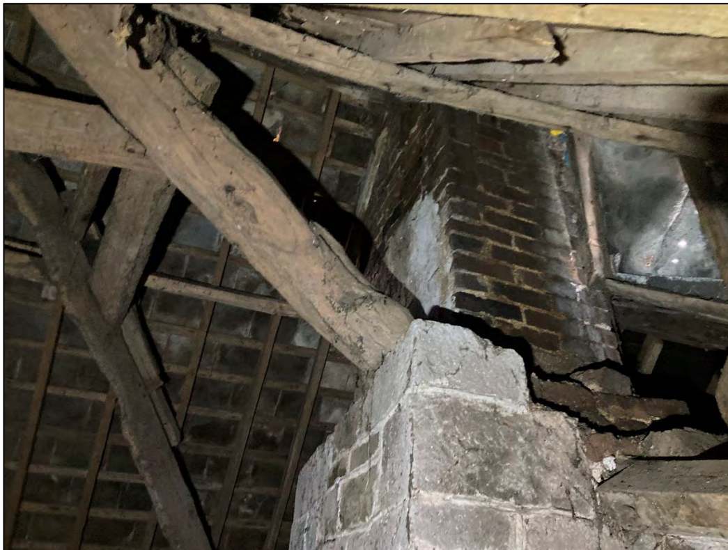
Figure 25: Chimney Stack at the eastern end of the Hall House Roof Space. View to the South.
