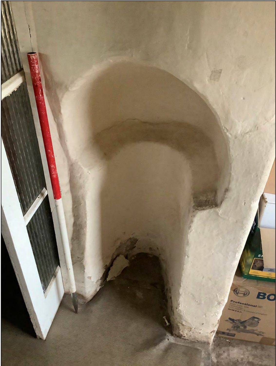
Figure 16: Cavity cut into former external wall that now separates Room 1 from the small extension to the south. Possibly the location of a Victorian bread oven.
