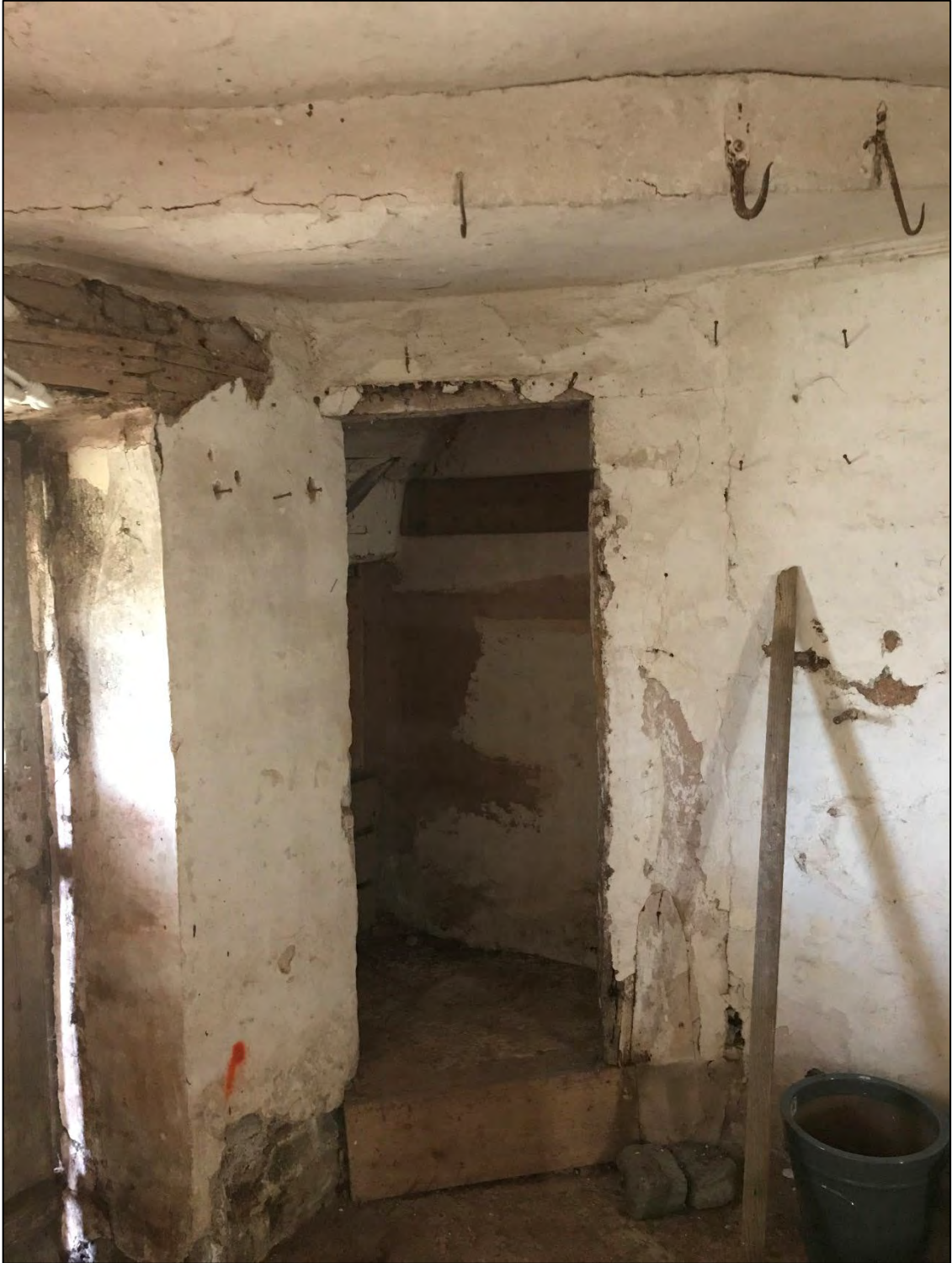
Figure 37: Storage space under the 17th century central staircase of the main hall house, taken from Room 8 in the southern block.
