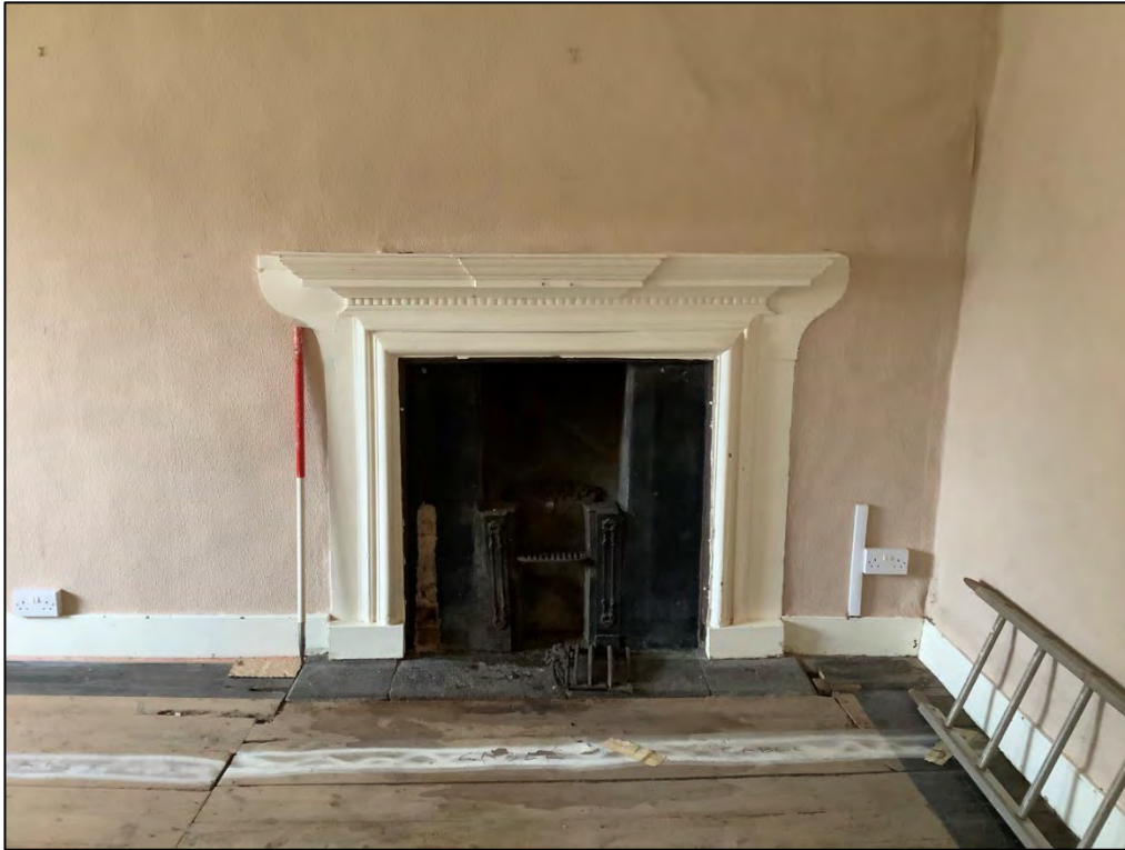
Figure 22: The 18th century fireplace surround with 19th century cast iron hearth within Room 7.
