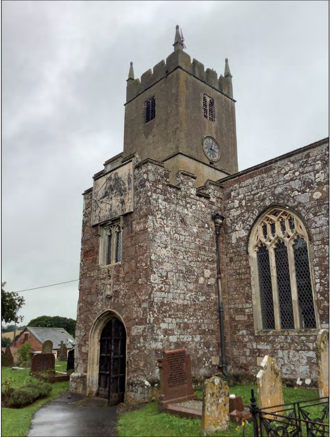
Figure 3: The Grade I Listed Church of St Matthew. View to the north west.
