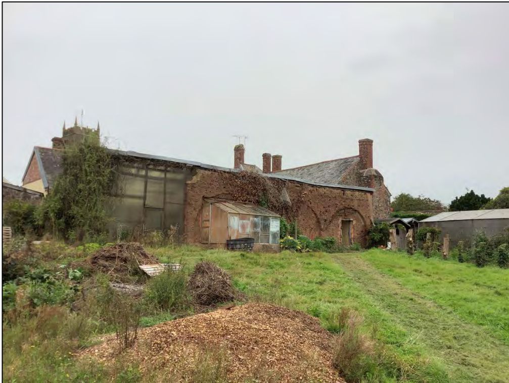
Figure 54: Cob wall to the rear of the southern stable block. View to the north east.
