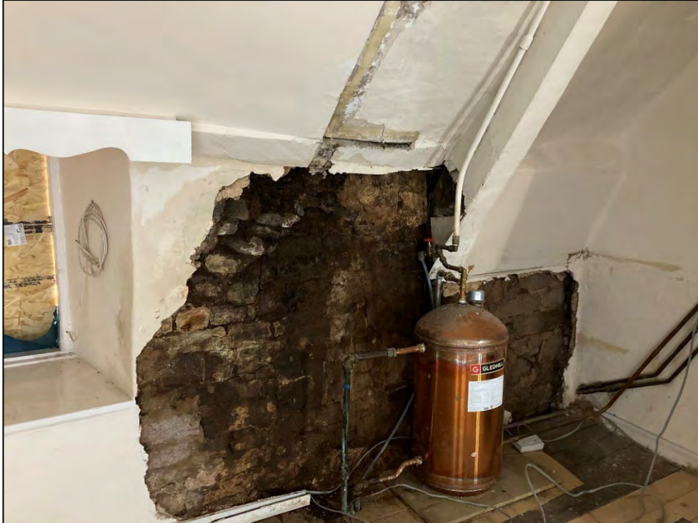
Figure 20: Damp damage to the fabric of the central stack and cob walls of Room 5 as a result of the installation of the slate roof in the 19th century. The oak true cruck truss (right) is still in a good state of preservation.
