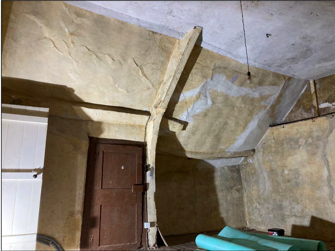
Figure 18: The cruck blade in the western end of the hall house first floor, Room 4. Beyond this the hall house has been extended from its original hipped roof to a gable end. The further timber beyond the cruck is of elm (right).
