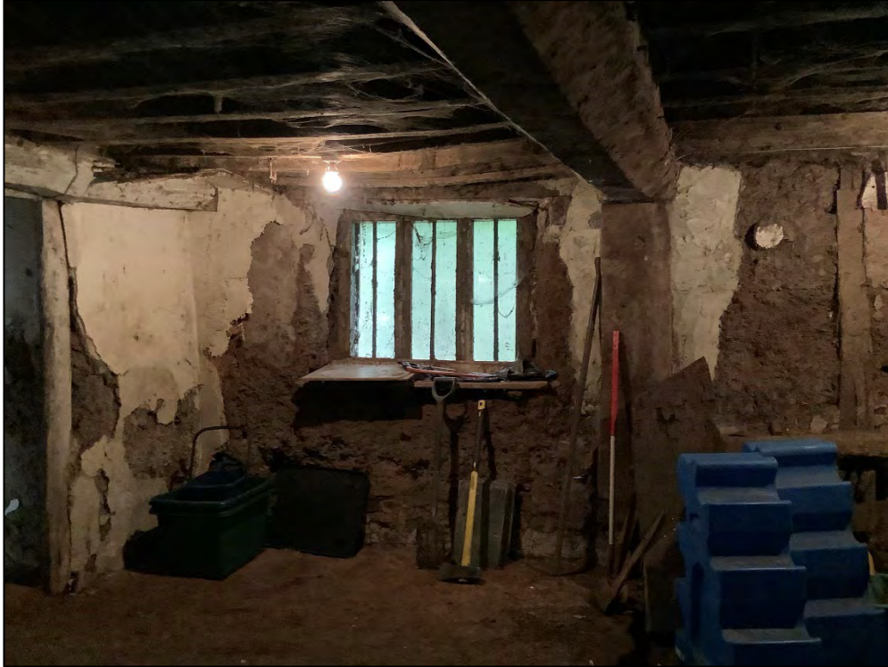
Figure 39: Possible original window opening. East of Room 9. The window has been re-framed and painted, however, the iron bars are thought to be original. The Horizontal oak tie beam is also thought to be original.
