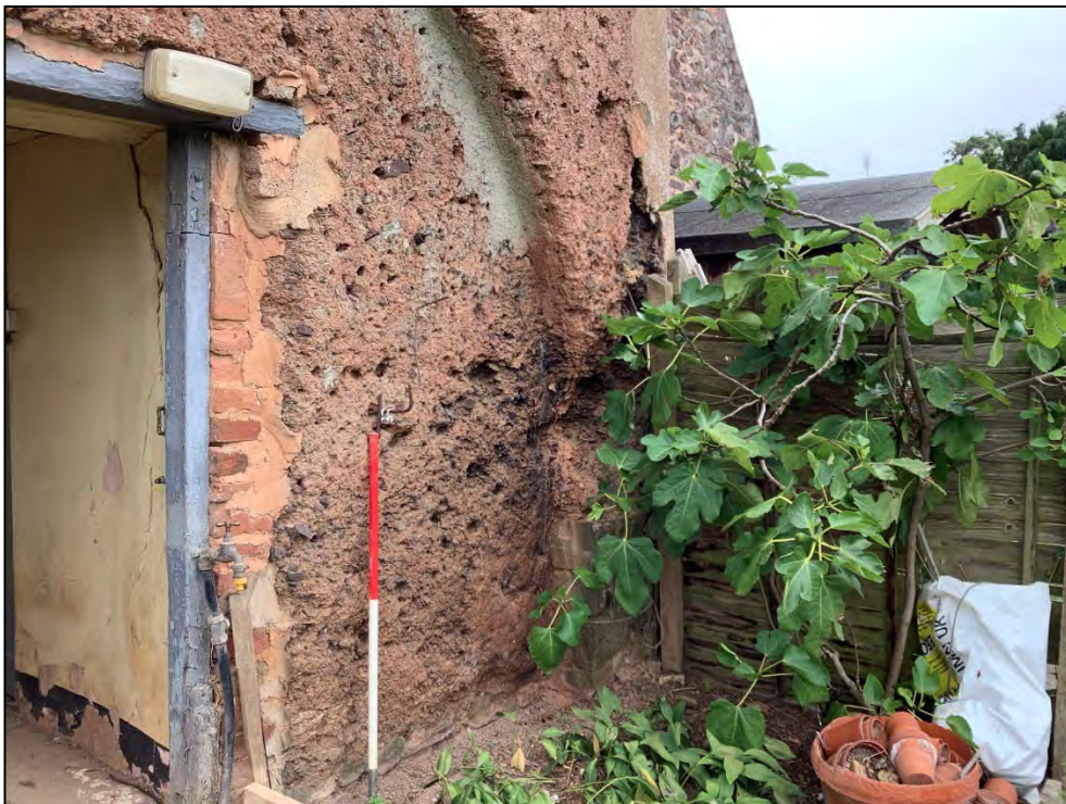
Figure 56: The remains of earthen plaster with the cob walls easternmost decorative arch. View to the north east.
