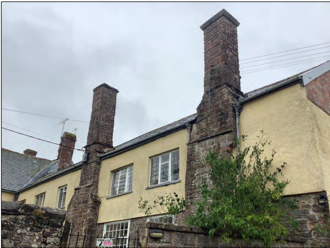
Figure 8: The two chimney stacks to the western end of the north facing elevation and the third stack to the east of the main block. View to the south east.
