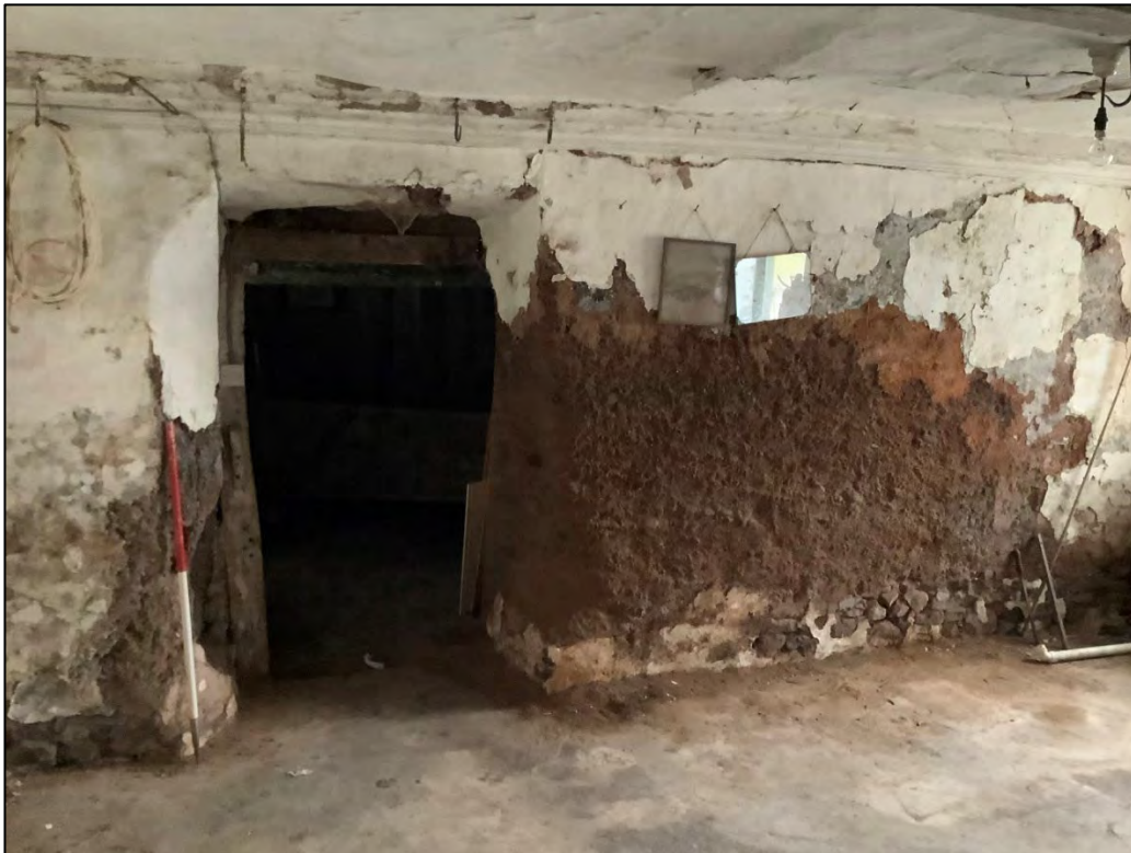
Figure 34: Cob wall dividing Room 8 with Room 9 to the south. Meat hooks can be seen within the oak crossbeams (top).
