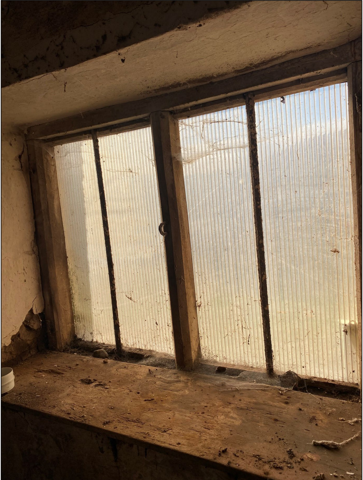
Photo 10: Historic window frame and ledge in Room 8 to be left in-situ, polycarbonate pane to be replaced with 12mm double glazing to provide warmth to the room and create a liveable space (Fig. 1, 3d)
