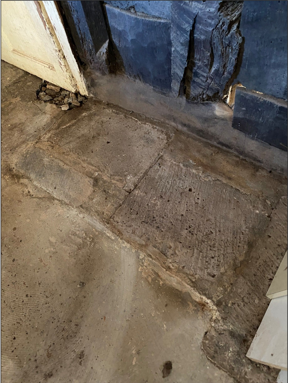
Photo 2: Historic Flagstone flooring in the south west corner of Room 1. To be left in-situ without impact (Fig. 1, 1)
