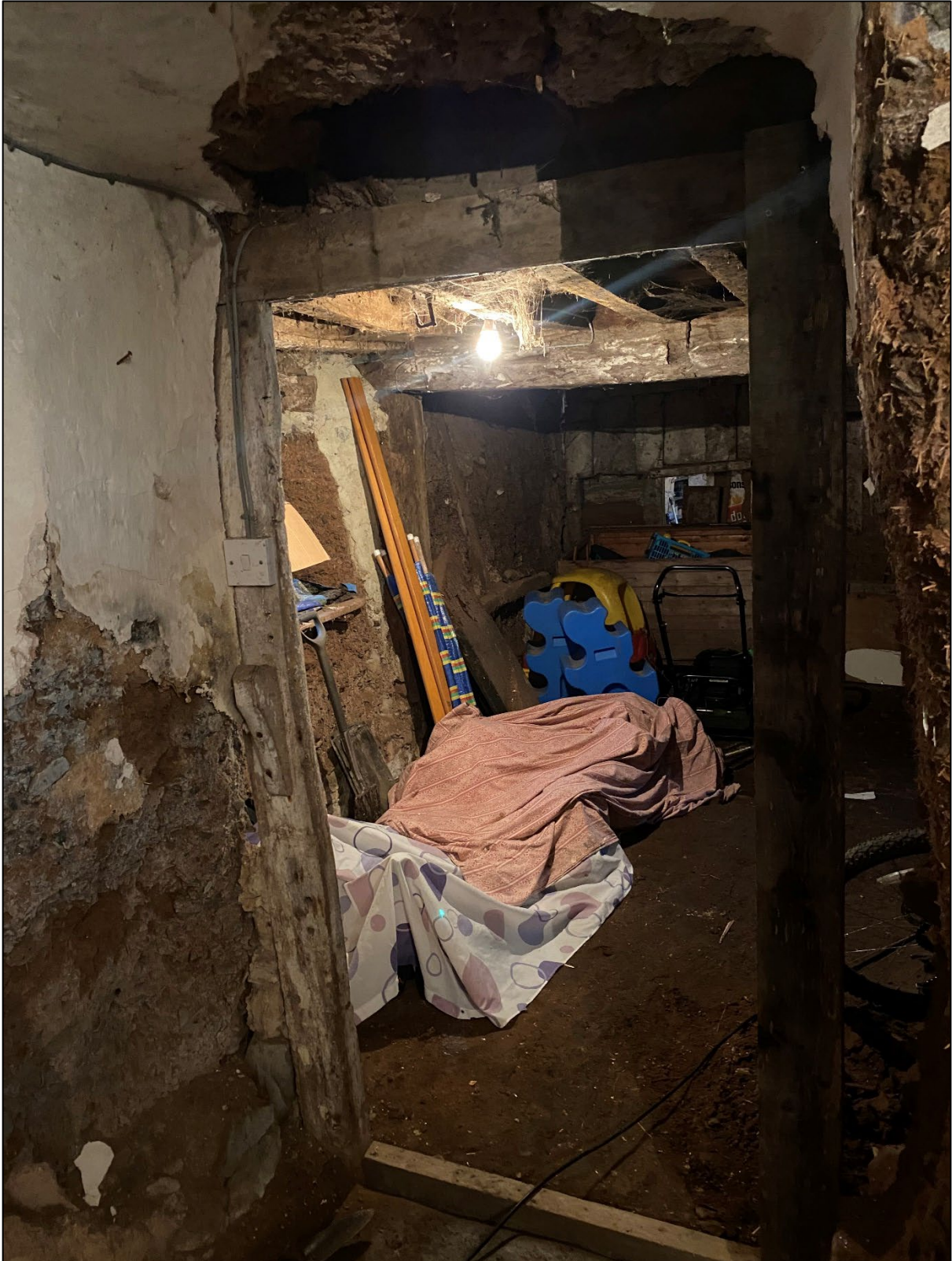
Photo 8: Existing oak doorframe between Rooms 8 and 9. The doorway is to be reinstated using a door respectful to the heritage of the house (Fig. 1, 3c)
