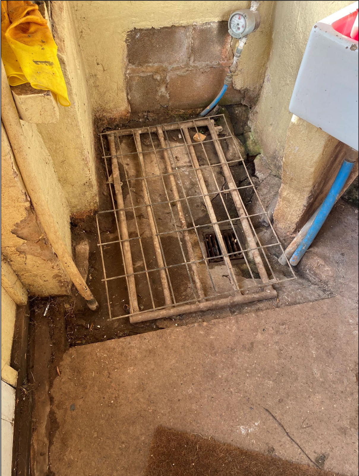
Photo 4: Drain within the rear porch to be covered or moved (Fig. 1, 2b)
