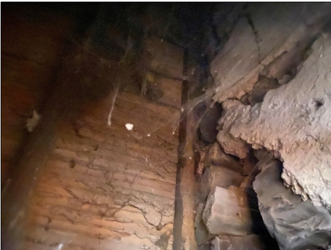
Photo 6: Cavity in the location of former doorway to be reinstated between Rooms 8 and 3 containing modern (20th century) woodwork (Fig. 1, 3a)
