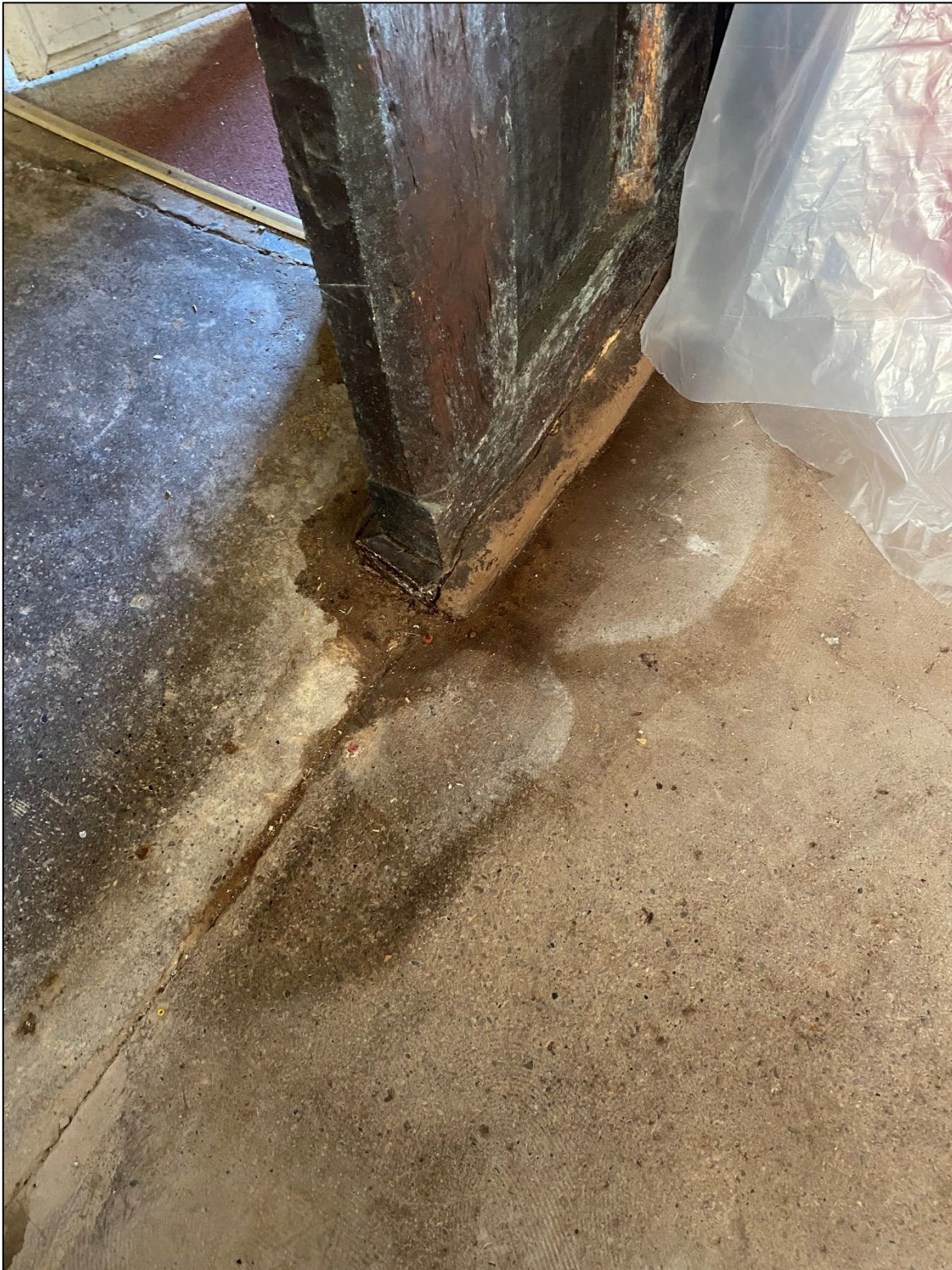
Photo 1: Damp coming through the modern concrete floor against the base of a 15th century oak plank-and-muntin screen (Fig. 1, 1)
