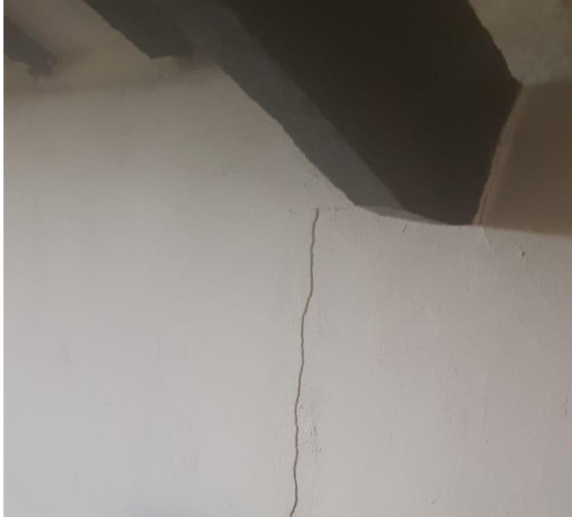
Above: Crack under truss bearing at first floor level.
