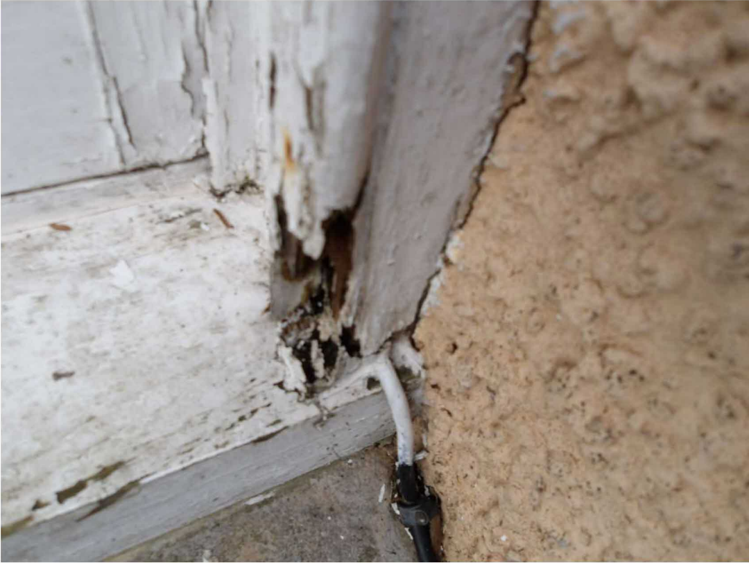
P2 – DAMAGE TO WINDOWS
