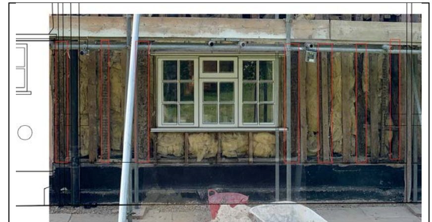
The kitchen window area (the area proposed for intervention) during the replacement render works last year. Original timbers are highlighted red.
