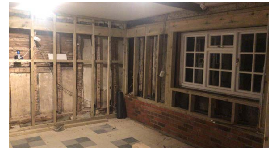
Taken during renovation works by the previous owners, the modern internal plinth is clearly visible.
