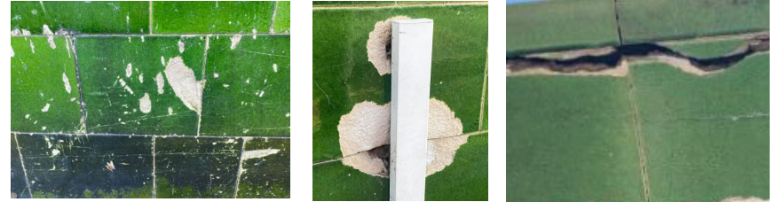
Annex H: Detailed Report of Tile Condition
