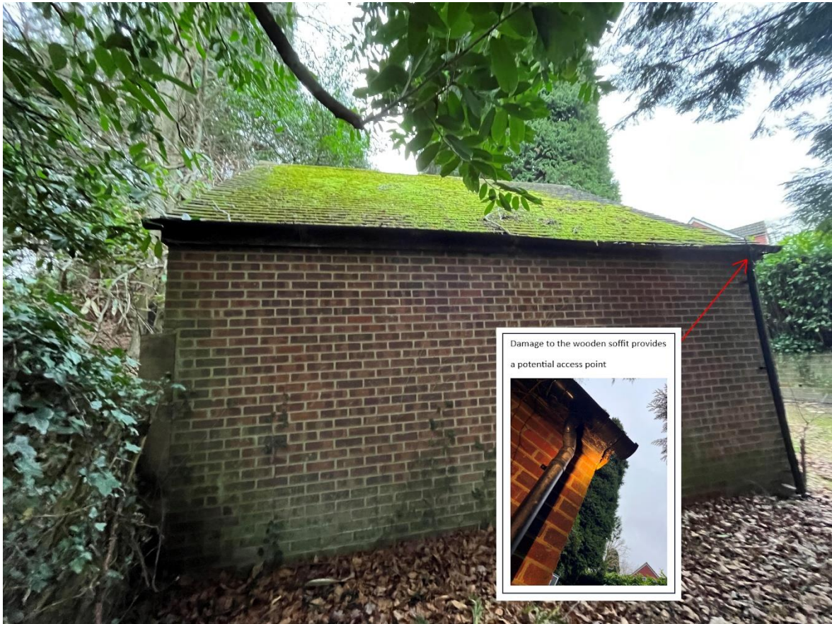
Image 4.3.1.2. Location of potential bat access points on the east elevation of the garage.
