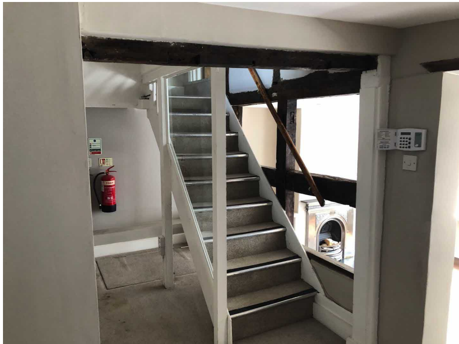
Modern Stair to be replaced and new stud walls retaining all timber framework
