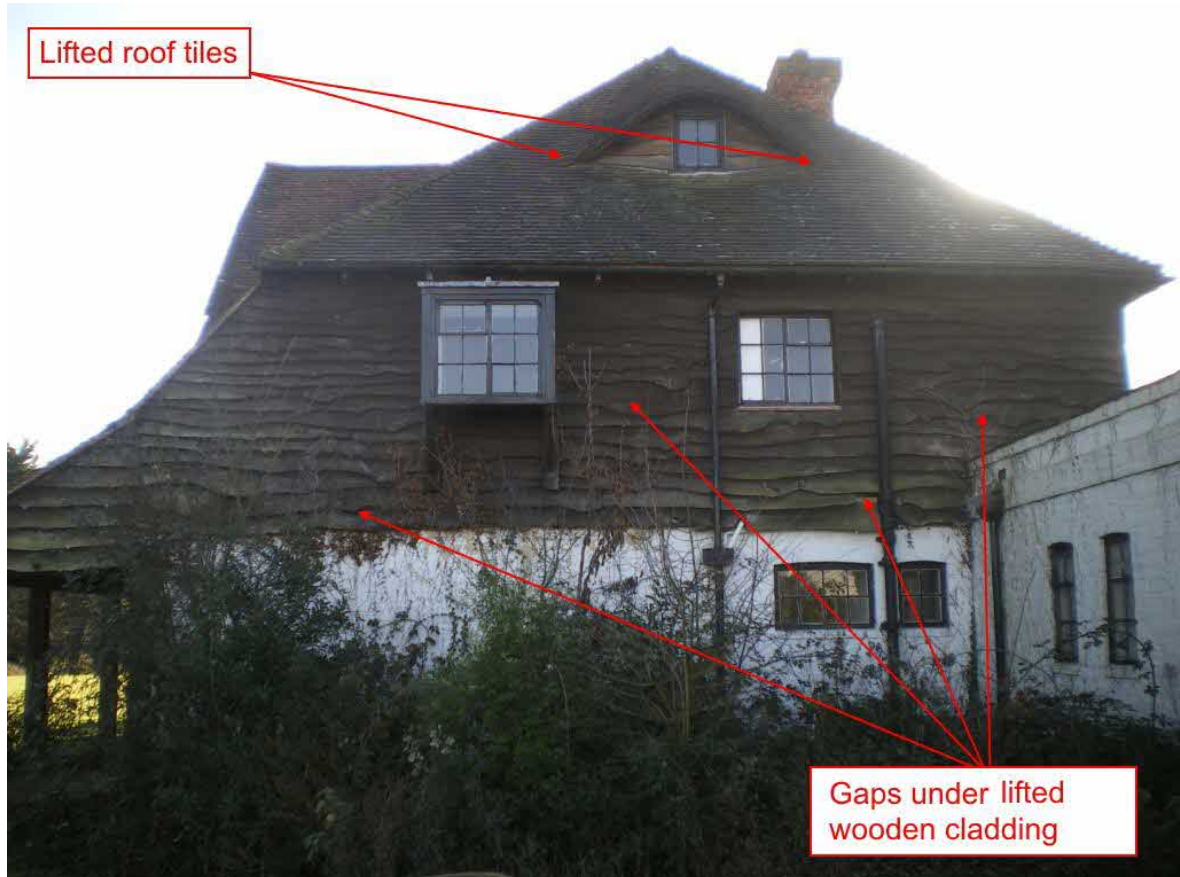
Image 4.3.1.1. Location of potential bat access points and potential exterior roof features on the north elevation of the house.
