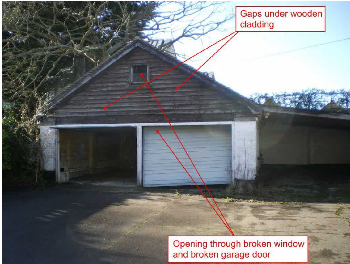
Image 4.3.1.5. Location of potential bat access points and potential exterior roof features on the east elevation of the garage.
