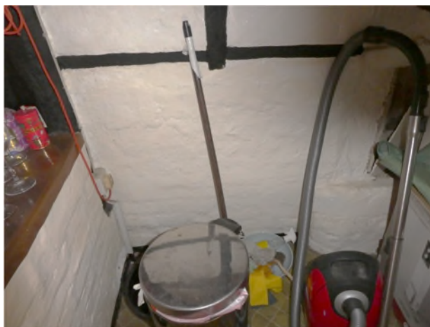
Figure 19: Position of a former door opening on the south-east side of Phase 1 (under the stairs in the kitchen)
