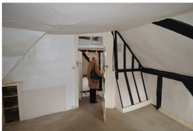
Figure 16: South-west side of bedroom 3 showing the position of the chimney breast (left) and later partition (right)
