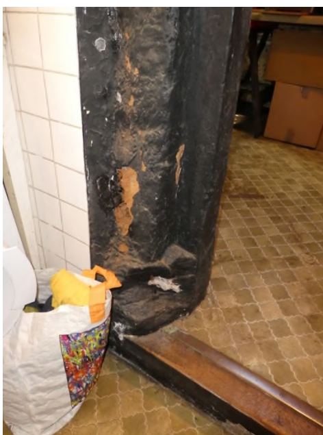
Figure 18: Sole plate and post in the opening between the front and rear kitchen
