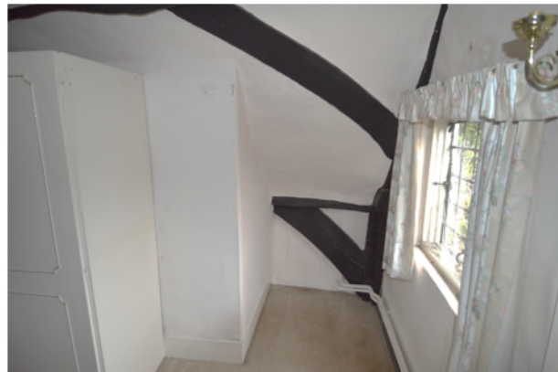
Figure 12: Curved head brace in the south corner of Phase 1
