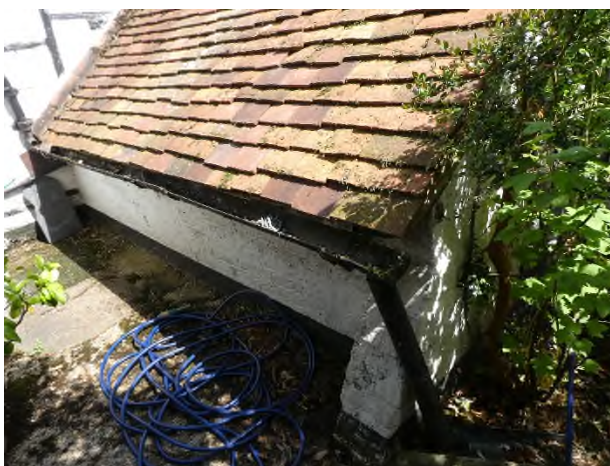
Figure 40: Brick outshut with a catslide roof to the rear of Old Timbers
