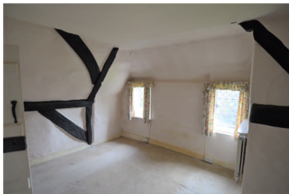
Figure 14: Cut tie beam associated with the Phase 3 extension
