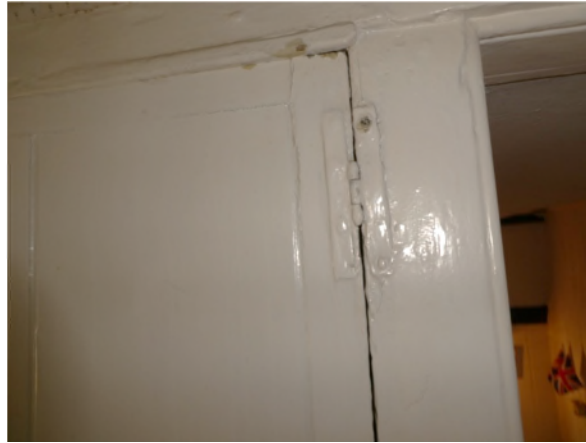
Figure 46: H-hinge to a late 18 th to early 19 th century cupboard in the bathroom
