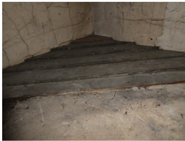
Figure 47: Weatherboard and plaster finishes to the central truss and skelting over the bathroom
