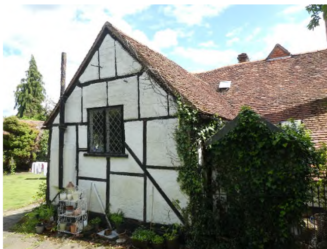
Figure 53: Rear elevation of the listed building showing the position of existing rooflights
