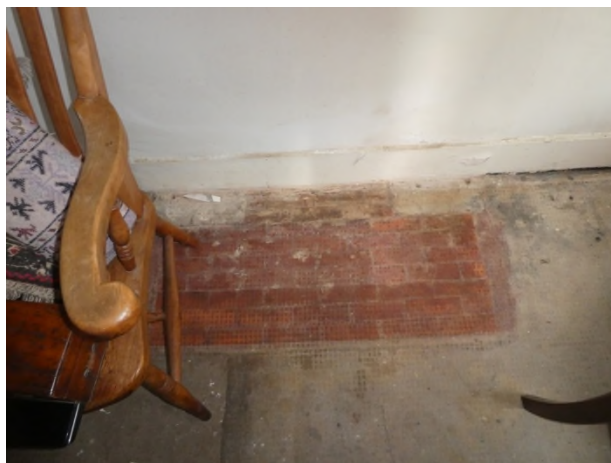
Figure 27: Evidence for a brick hearth in front of the chimney breast in the dining room
