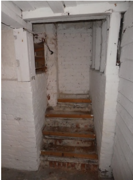
Figure 57: Steps leading to a blocked opening to the cellar from the entrance hall
