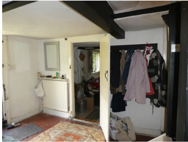
Figure 20: Partition wall on the south-east side of the entrance hall from the garden marks the probable position of an axial beam
