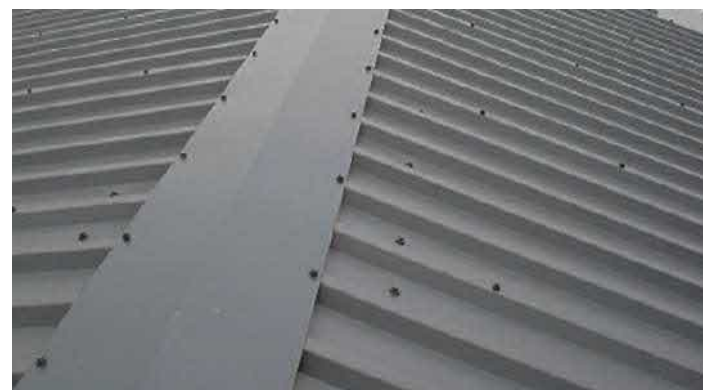
Precoated metal roof with matching flashing
