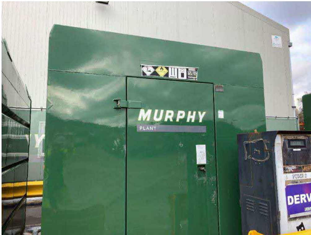
Photograph 3: Diesel is stored in 3 6-7000l tanks with inbuilt bunds. They are locked at all times.
