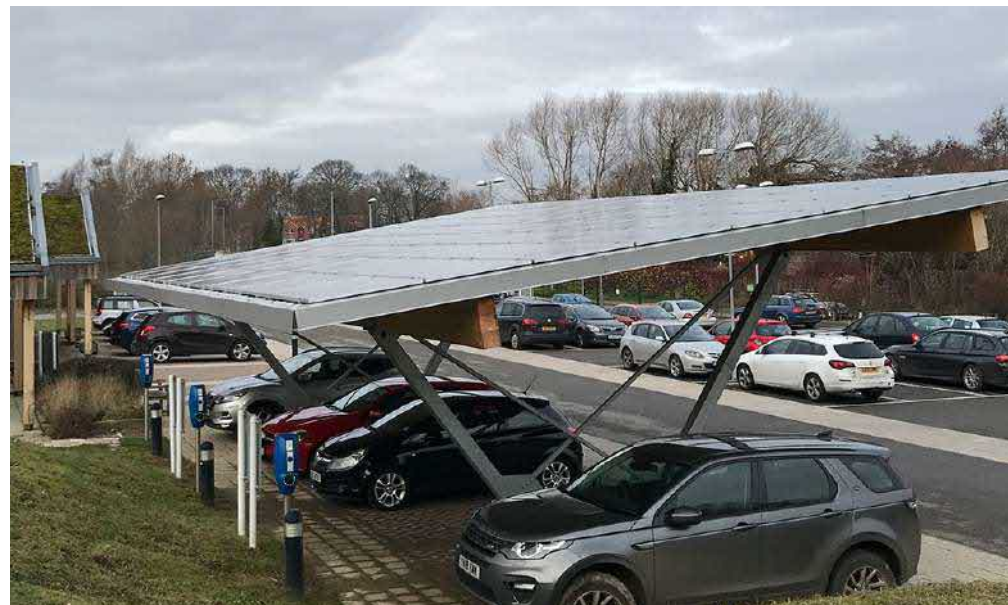
Reference image: Photovoltaic Carport
