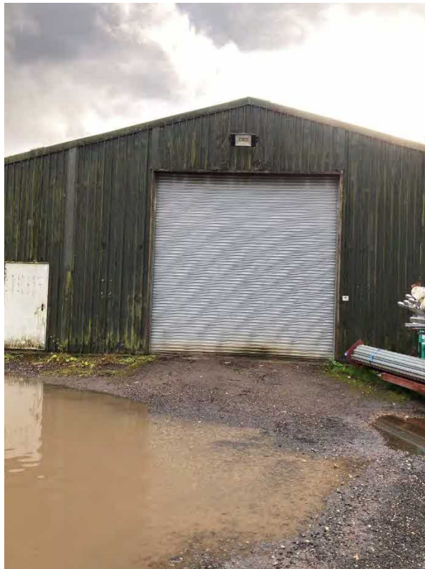
Photograph 10 –Gaps under metal sheeting of B10
