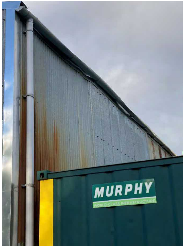
Photograph 9 –Gaps under metal sheeting of B8
