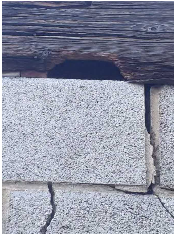
Photograph 8 –Soffit gaps in B5 and cracked breeze block
