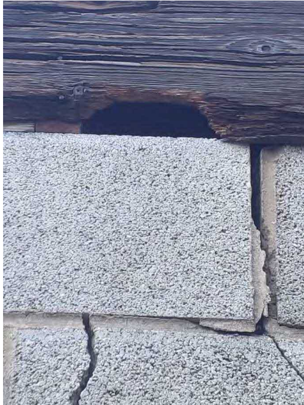
Photograph 7 –Soffit gaps and cracked breeze block in B5
