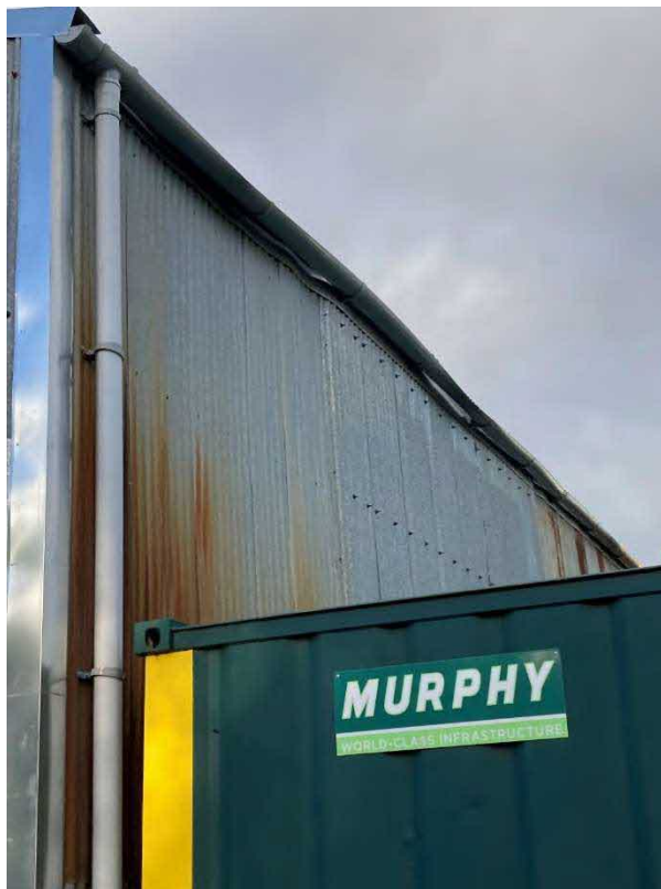
Photograph 8 –Gaps under metal sheeting of B8
