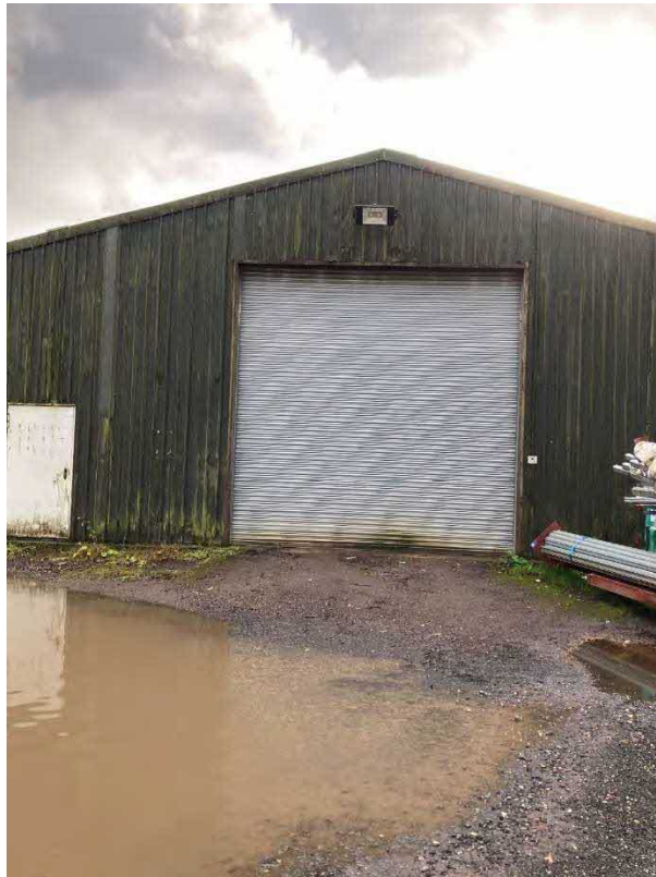
Photograph 9 – Gaps under metal sheeting of B10
