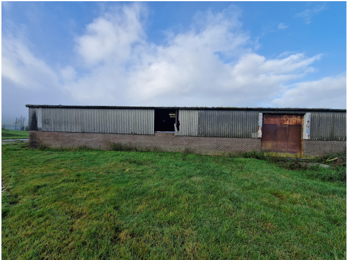
Above: View of the existing, east, barn elevation showing broken/missing sheet cladding, heavily rusted doors, areas of damp and vegetation growing out of the gutters
