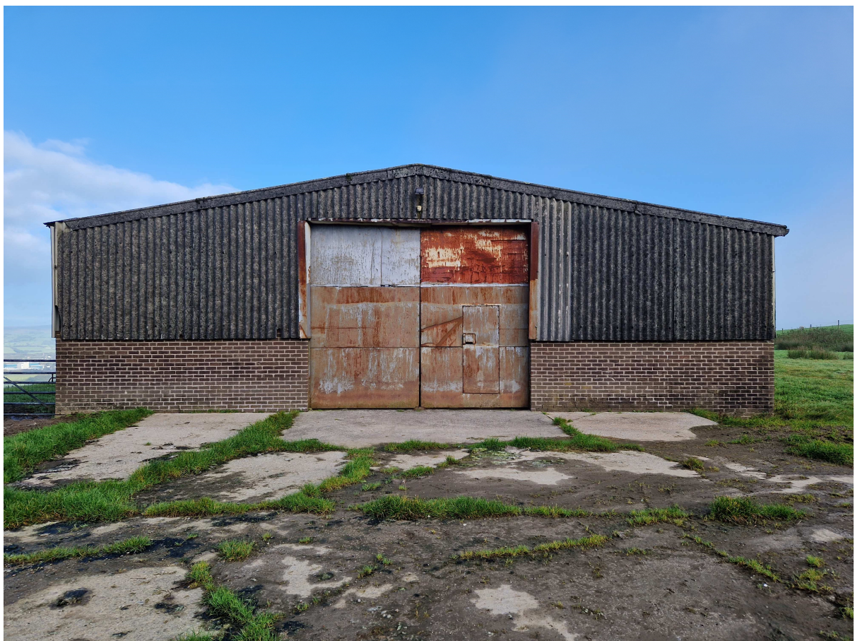
Above: View of the existing, south, barn elevation showing rusted doors and weathered cladding
