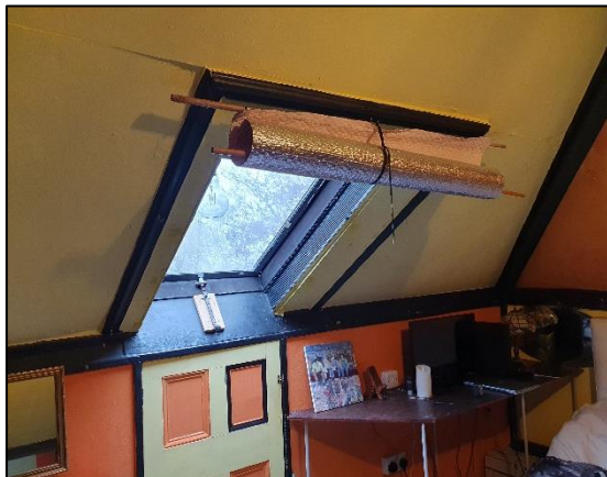
Figure 5: Bedroom in roof space – no roof void.
