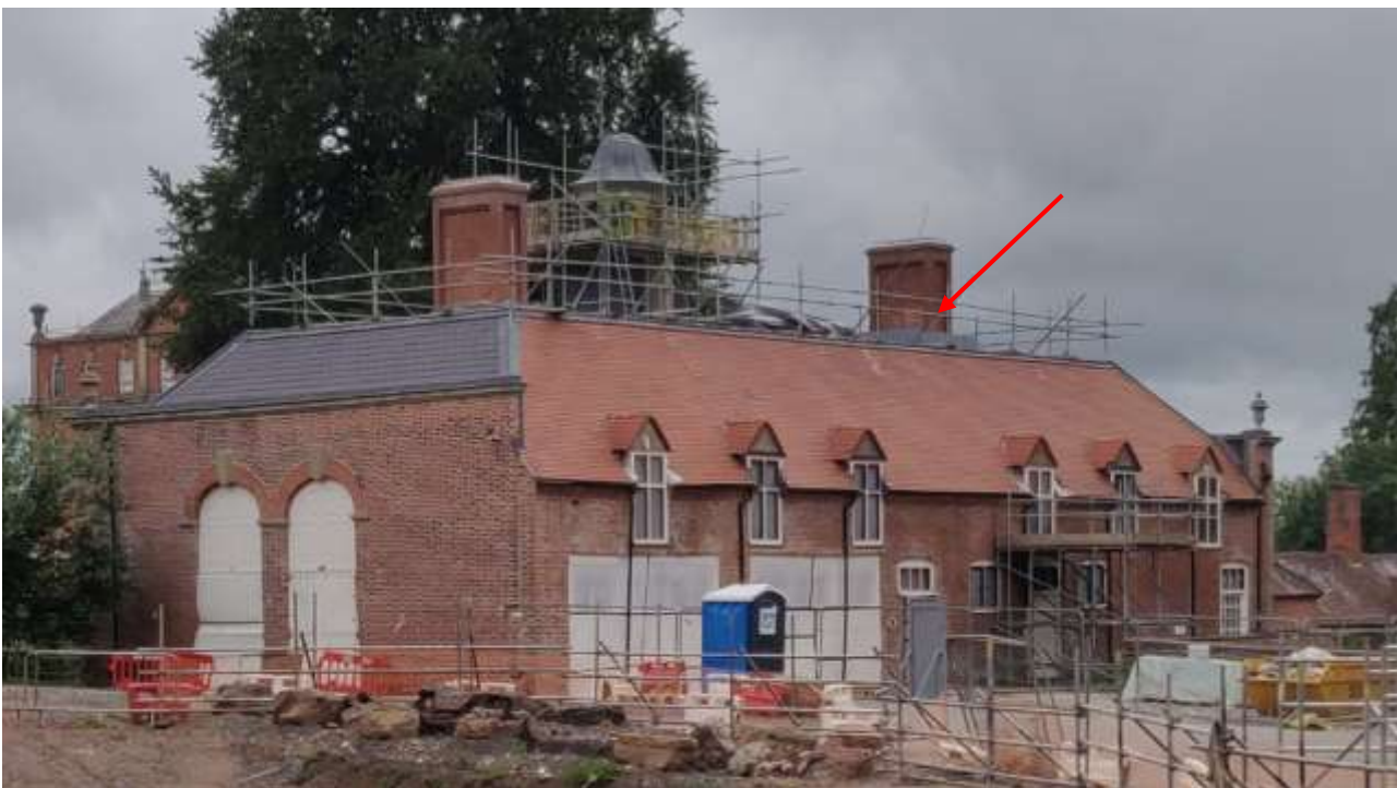
Fig. 2: View from the east end of the Spa Barn (red arrow points towards roof ducts)
