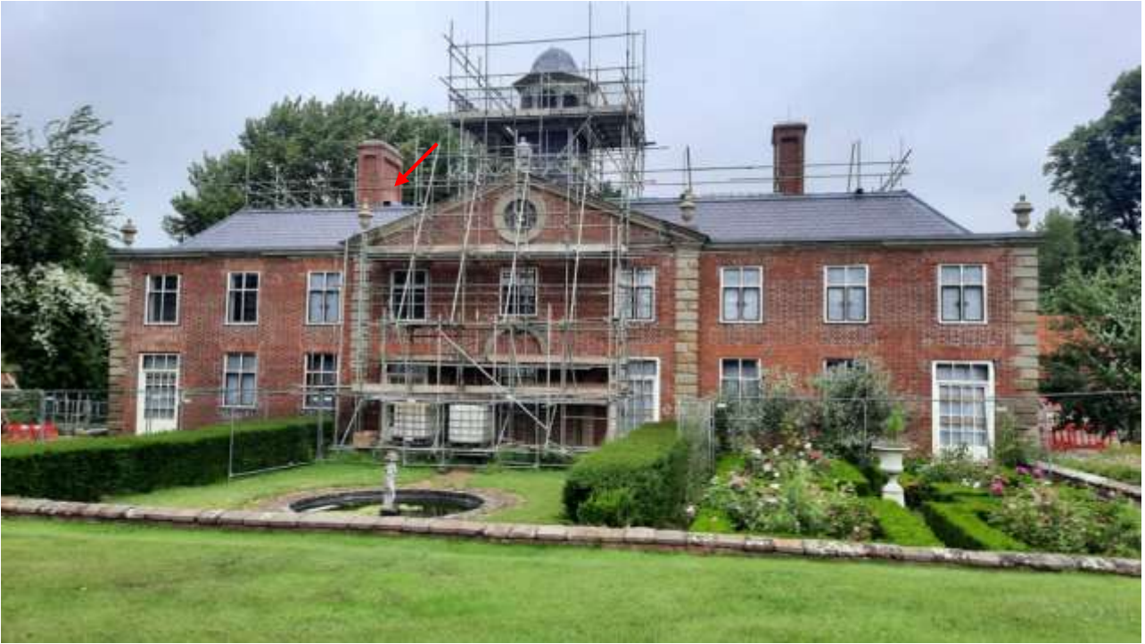
Fig. 3: View from the East Drive, south of the Coach House (red arrow points towards roof ducts)
