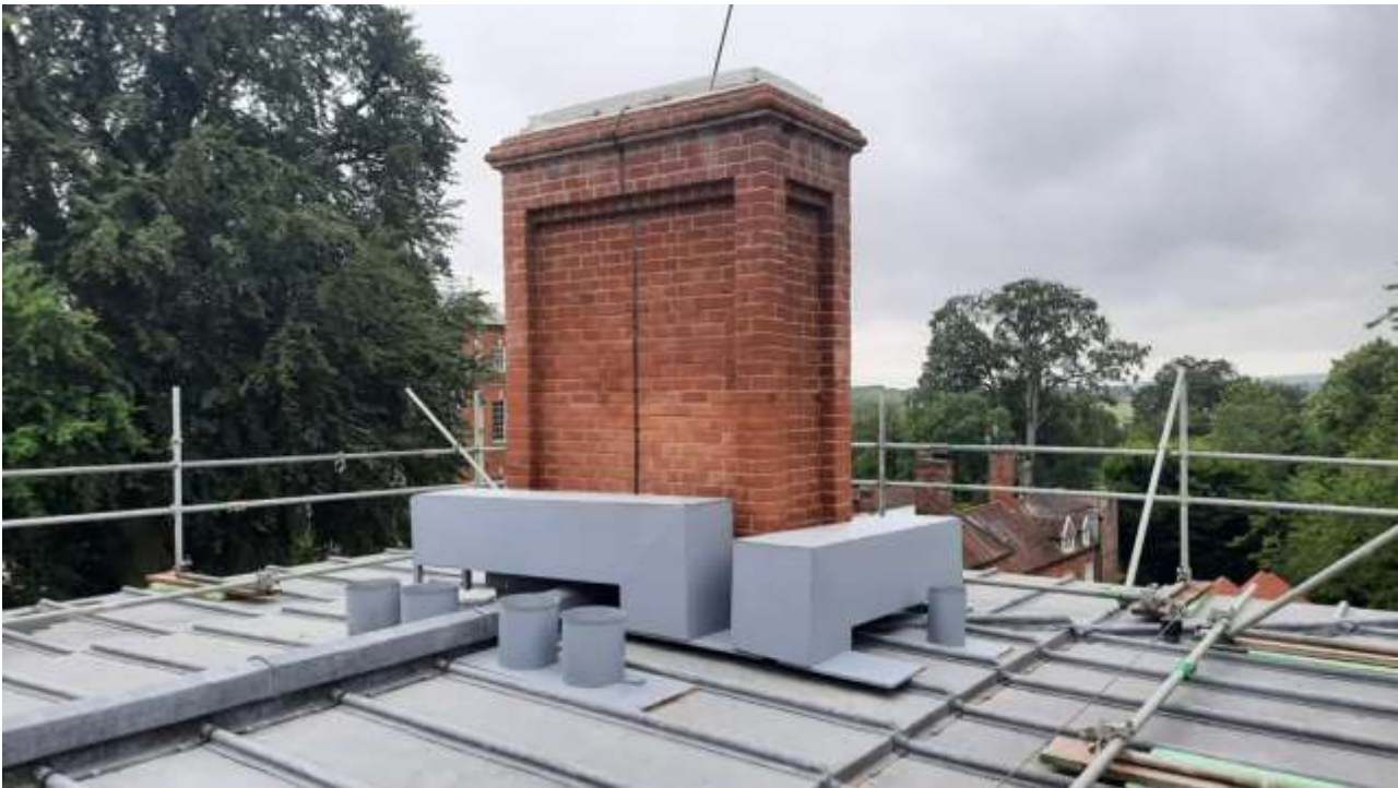
Fig. 1: Roof penetrations mock-up including the rectangular Service Kitchen intake and extract ducts
