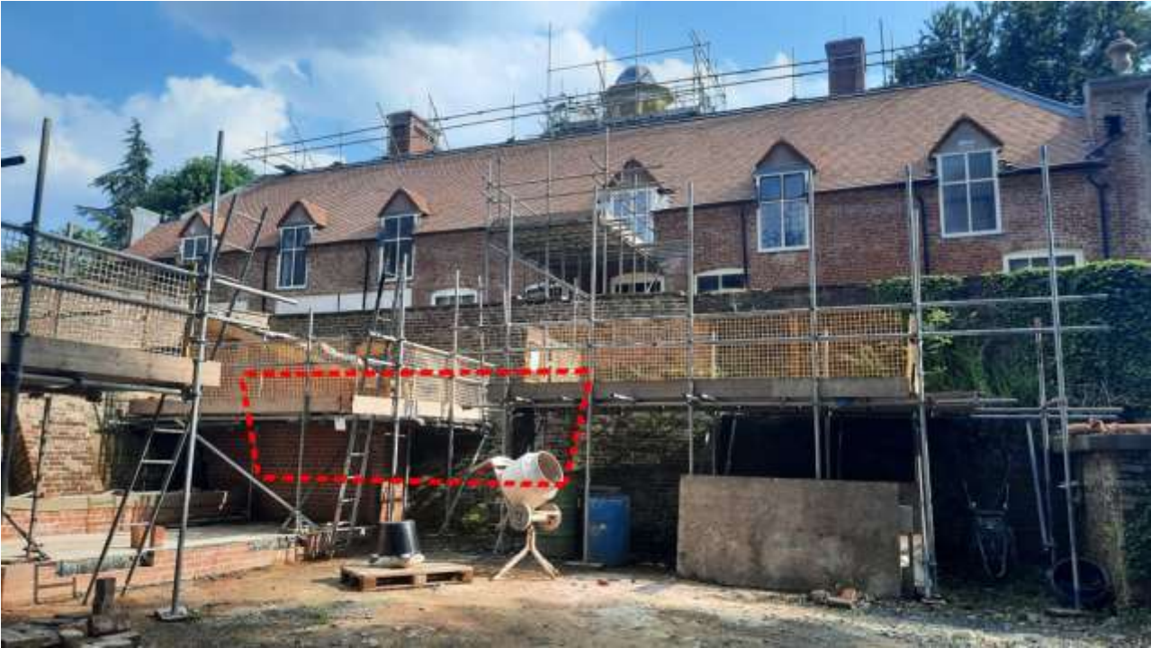
Fig. 5: View looking south from the Condenser Enclosure courtyard, with the proposed area of retaining wall for terminating the ducts shown dashed in red
