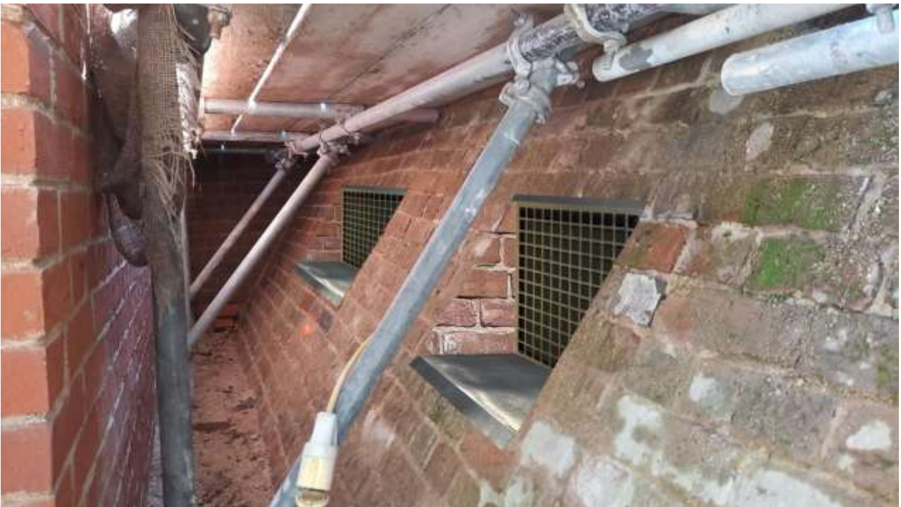
Fig. 6: Photoshopped image showing how the duct terminations in the base of the retaining wall are proposed to look, to the south of the Condenser Enclosure (the scaffolding currently visible will be removed on completion of the Enclosure)
