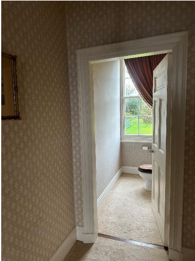
FIG 19 – Photograph of door to be closed up from lobby of dressing room (S Pemble)
