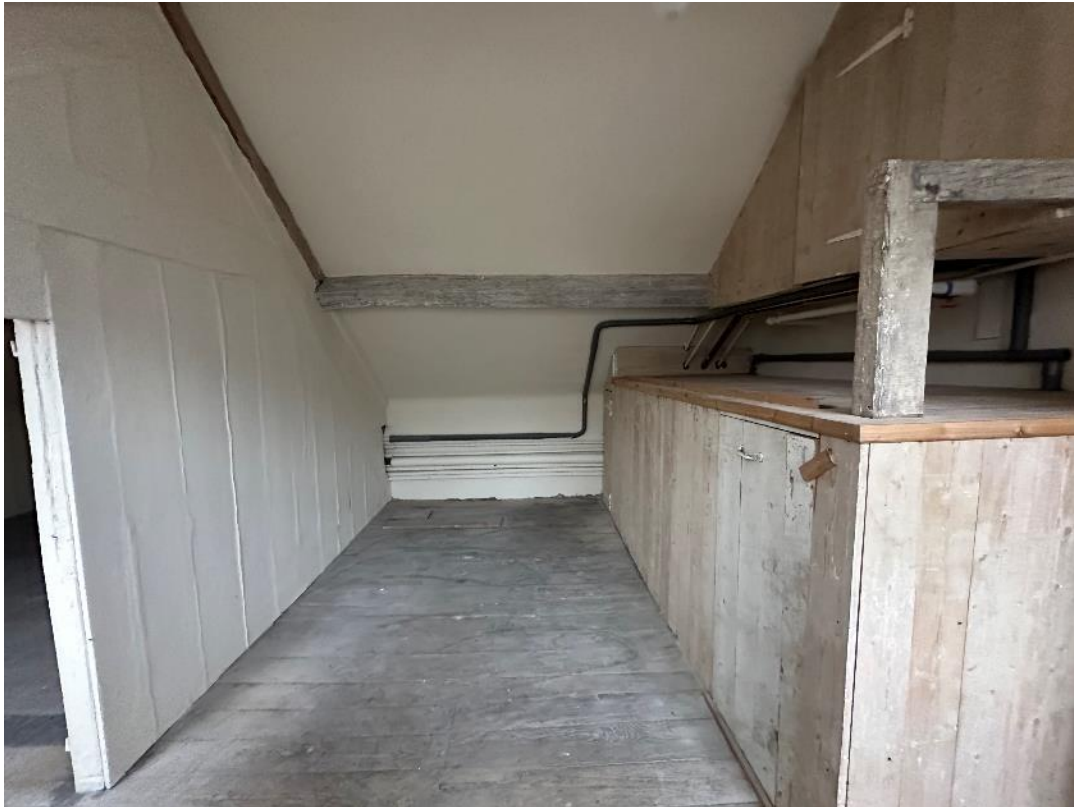
FIG 13 – Photograph showing area for attic floor bathroom – tanks to be removed (S Pemble)
