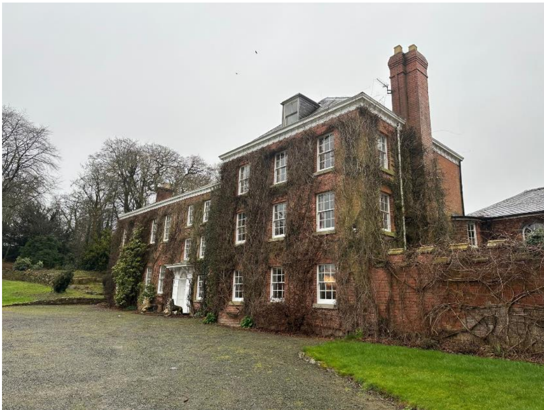
FIG 8 – Photograph from north approach of the main elevation (note soil pipe not visible)
