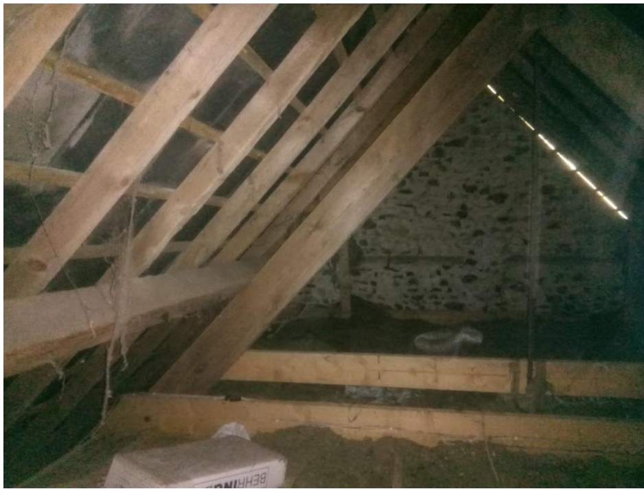
Current loft space above the proposed FF bedroom. The ceiling of which has now been removed.
