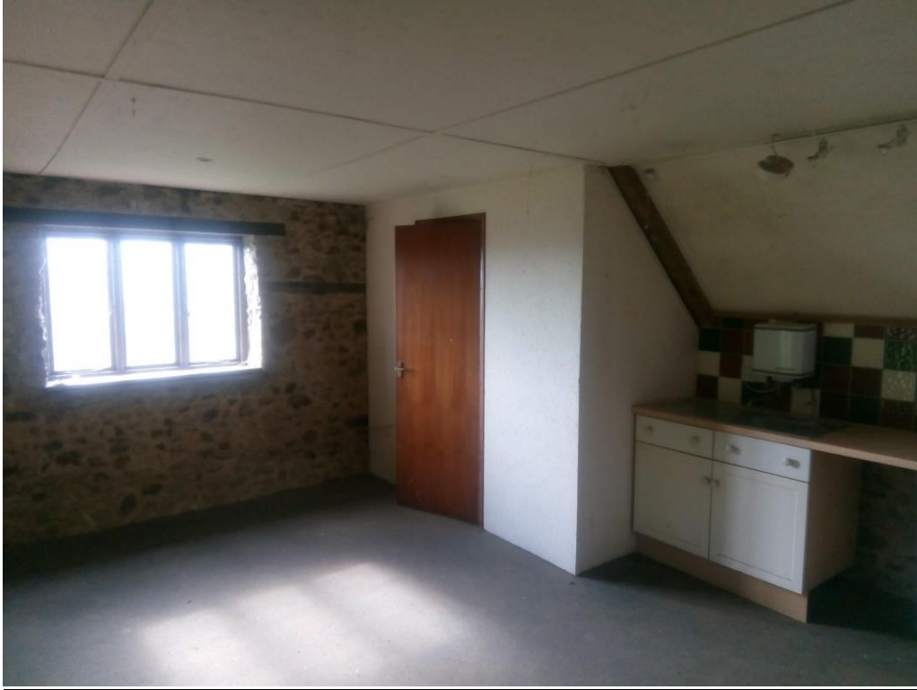
“Existing Kitchen & W.C. door” on First floor of Area looking South; now removed and forming part of a recent “retrospective” LBC application.
