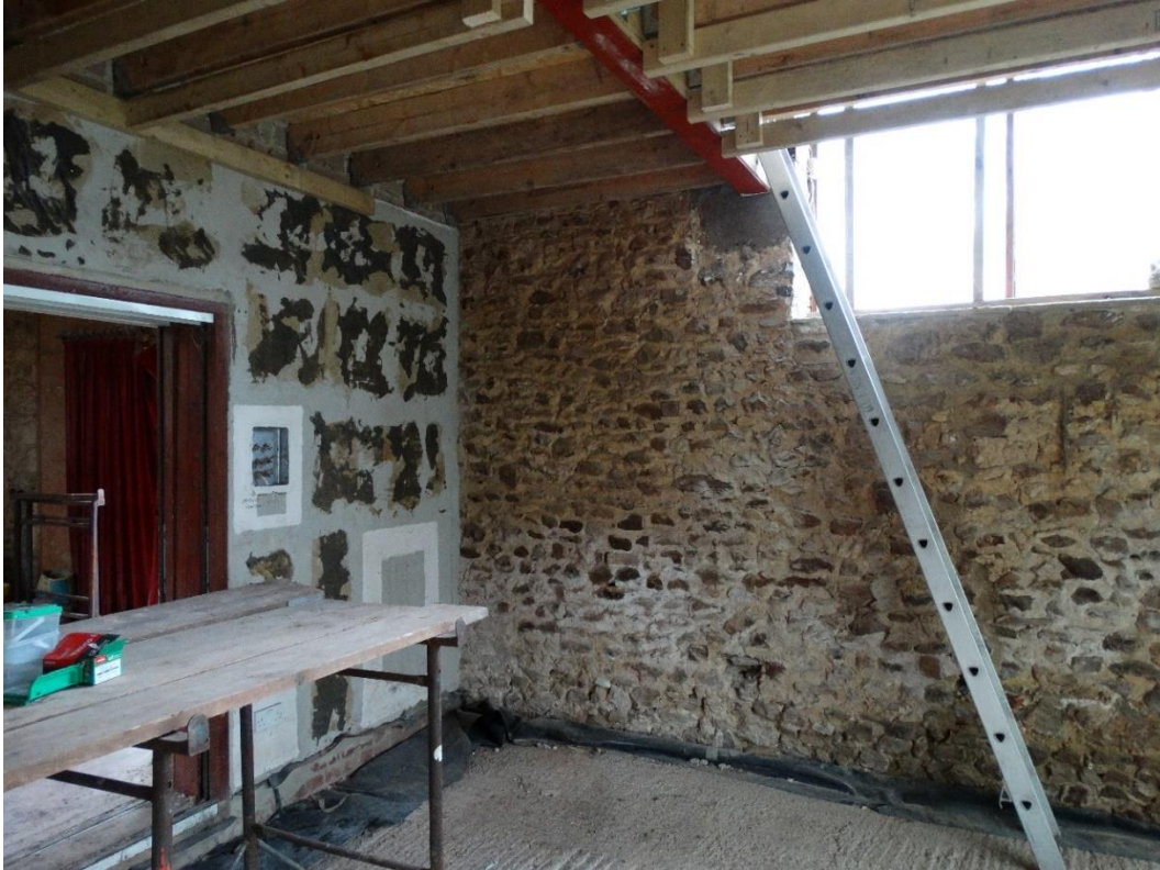
Current view of the east wall/ window aperture with the staircase removed & undersized softwood floor beams replaced with steel as recent “retrospective” application.
