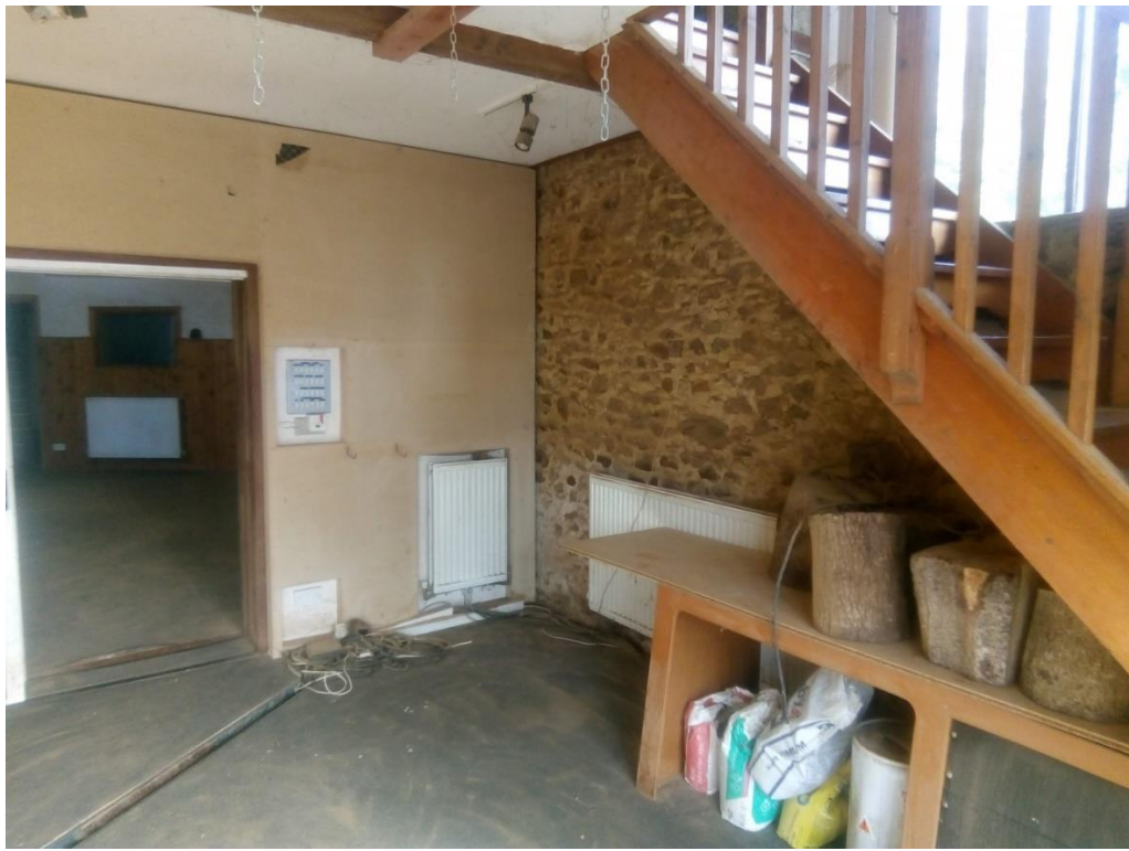
“Existing” Ground Floor of Area with staircase now removed forming part of a recent “retrospective application.
