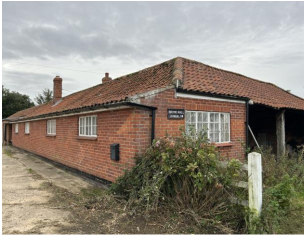
Image of dilapidated building to be renovated and extended
