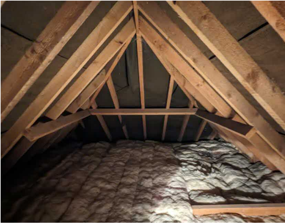
Figure 2. View of the loft space with this section the area that will be extended slightly (taken March, 2024).
