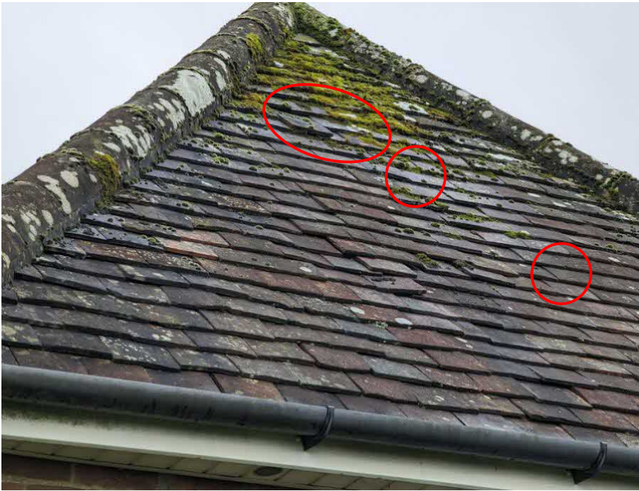
Figure 3. Additional PRFs noted where the existing flat roof section ties into the roof (this area will be impacted upon by the
