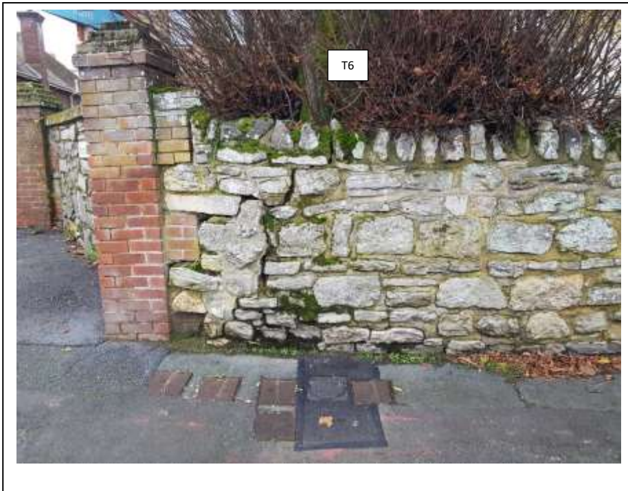
View of damage adjacent to T6
