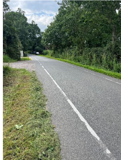
Photographs 4 and 5: Pauletts Lane Conditions
