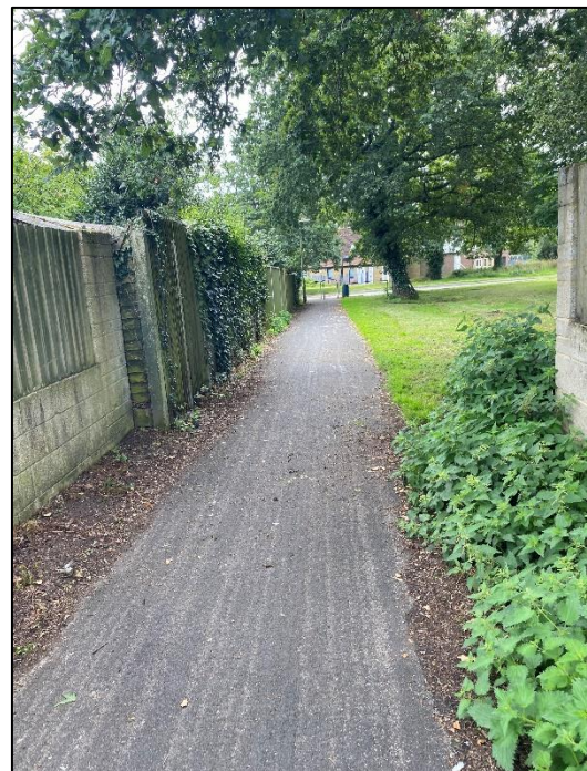
Photograph 13: Conditions on footpath from Calmore Road to Calmore Drive
